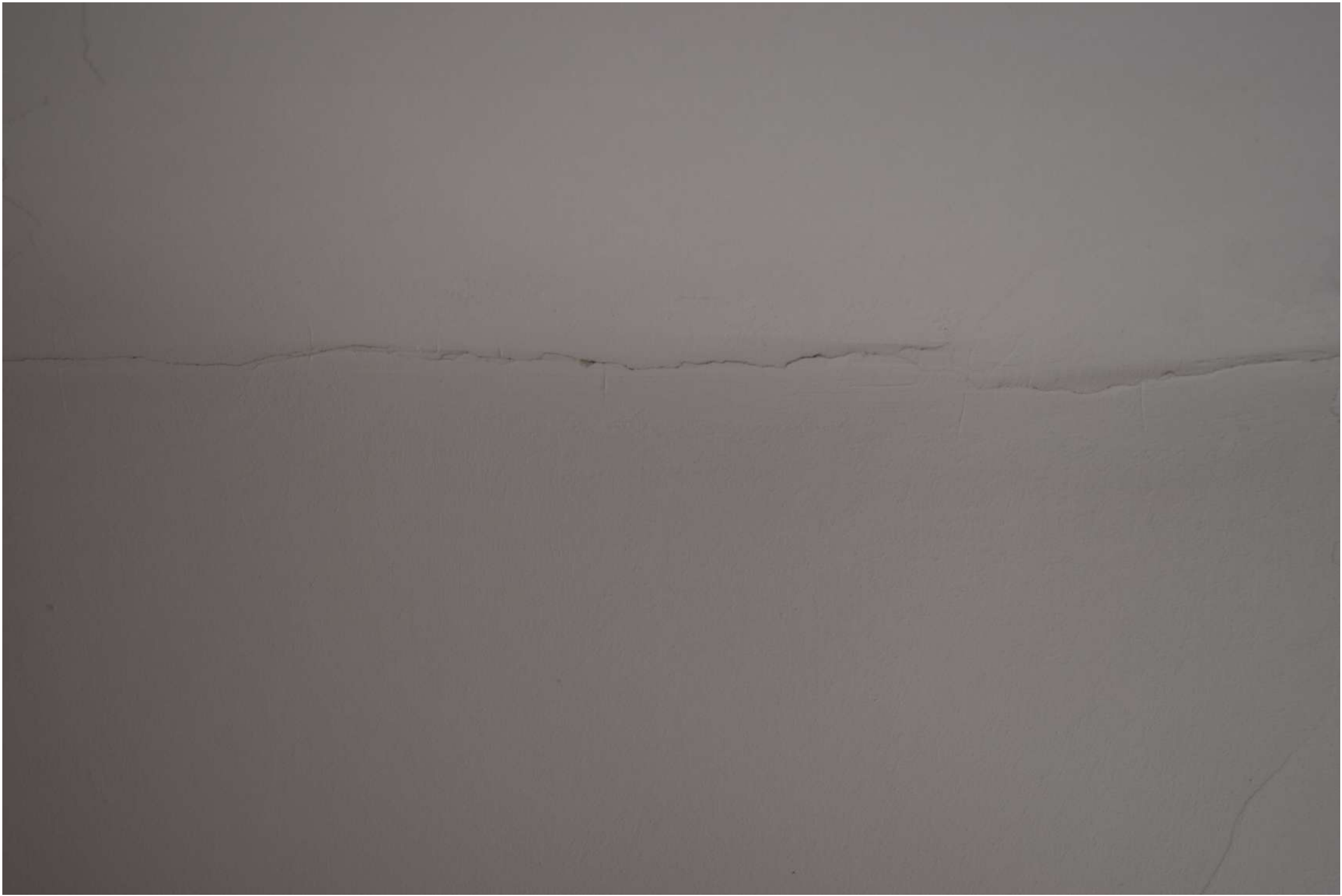
Plate 6 A condition issue: Detailed image of surface cracks beneath the main staircase, necessitating remedial repair works.
