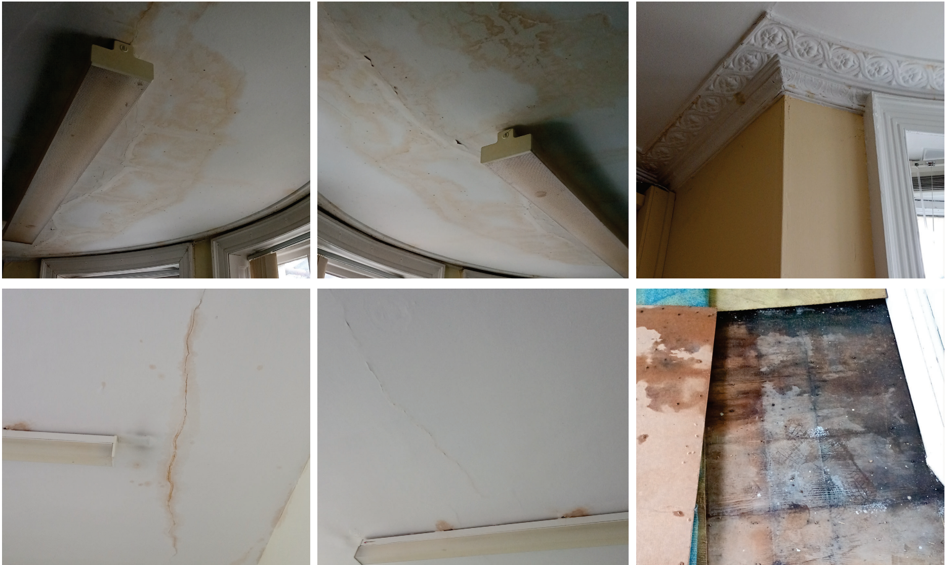
Plate 2: The internal damage is noticeable comparative to the previous images, on the first floor and ground floor due to lead theft on the roof.
