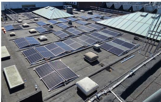
Typical Ballasted PV Installation
