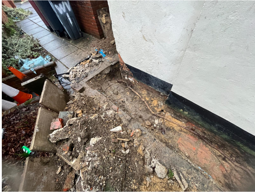
Plate 4 – historic original level (red quarry tiles) showing roots over this level that have grown in the sub-base of the paving slabs.
