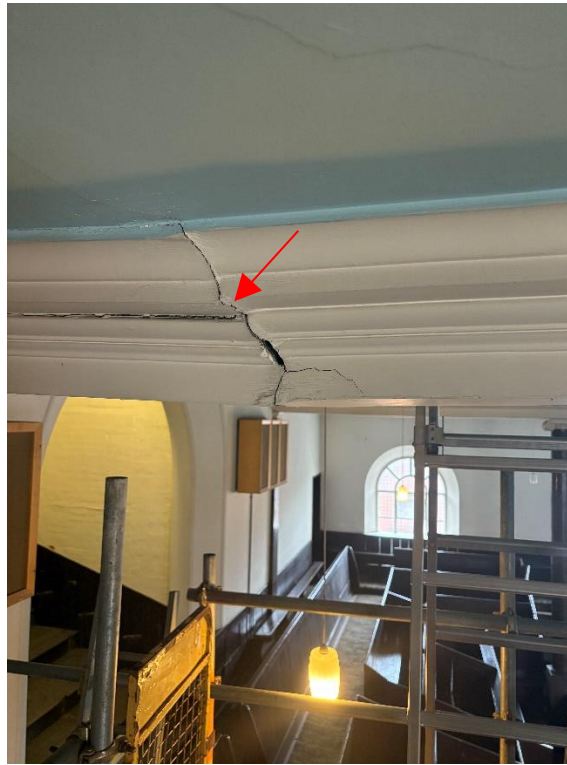
Figure 8. Fracture in timber beam to the south end of the church.
