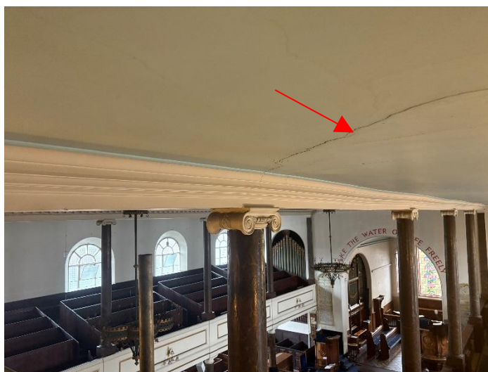
Figure 7. Minor cracking to ceiling over the nave.
