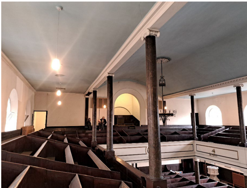
Photo 4 Looking towards failed beam from north end of church
