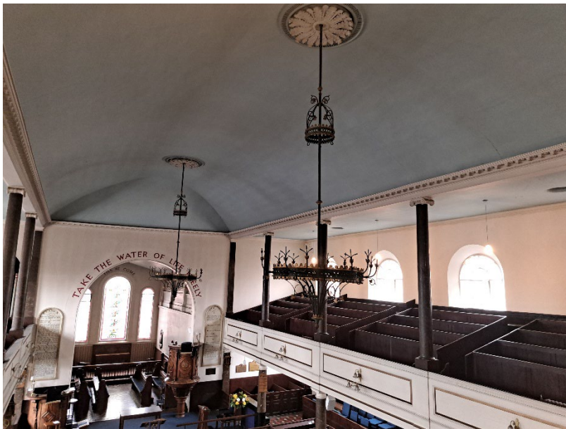
Photo 5 and 6 Repair area needed following a rwp leak
