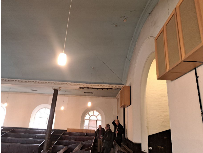
Photo 3 Area of redecoration needed looking towards failed beam
