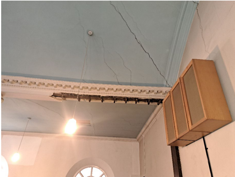
Photo 2 and 3 Failed Beam over Church Nave
