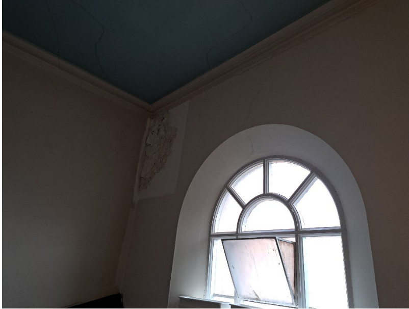
Photo 7 Location of plaster repair needed following rwp leak.
