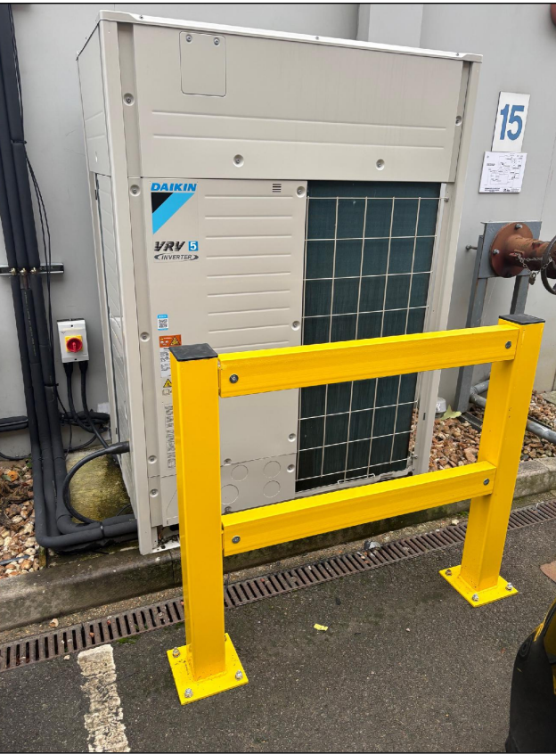
Vehicle Protection Barrier
