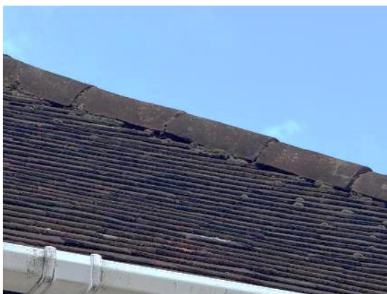
Photograph 7. Hip tiles with spalled mortar
