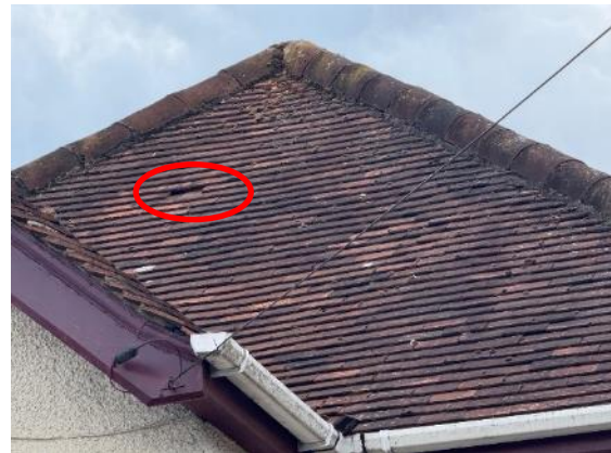
Photograph 2. Roof tiles with gaps between tiles
