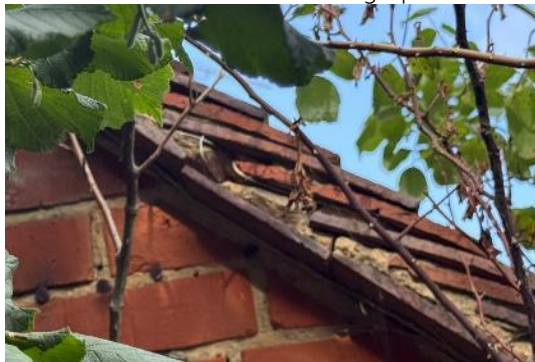
Photograph 21. Close-up of spalled verge mortar
