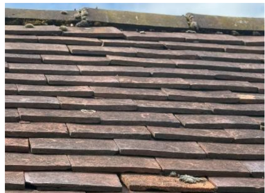
Photograph 18. Close-up of lifted tiles
