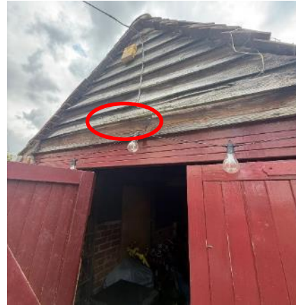
Photograph 16. Close-up of lifted and exposed cladding
