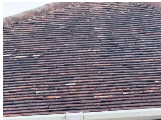
Photograph 6. Roof tiles with minor lifts
