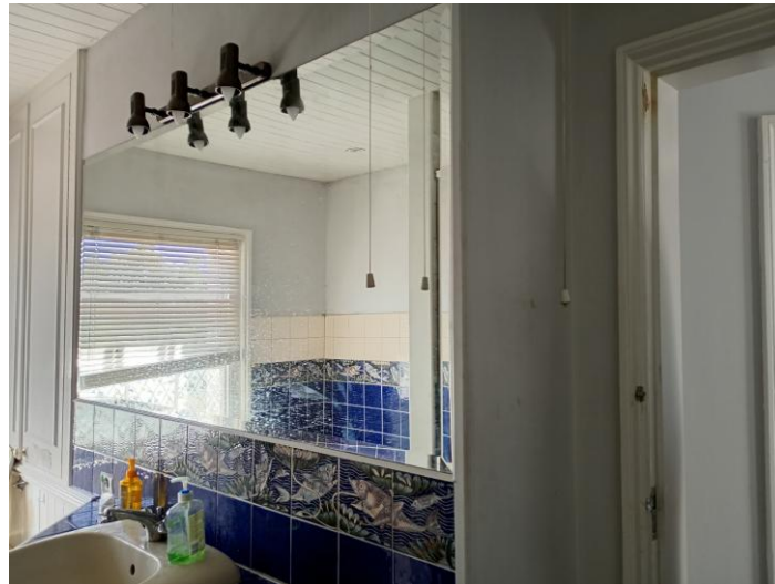
Figure 9: There is a chimney behind this bathroom cabinet
