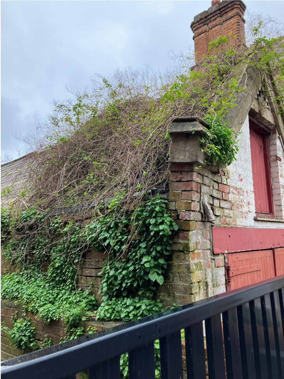
The damage to the NW corner
