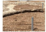
Example of air vent to brown roof
