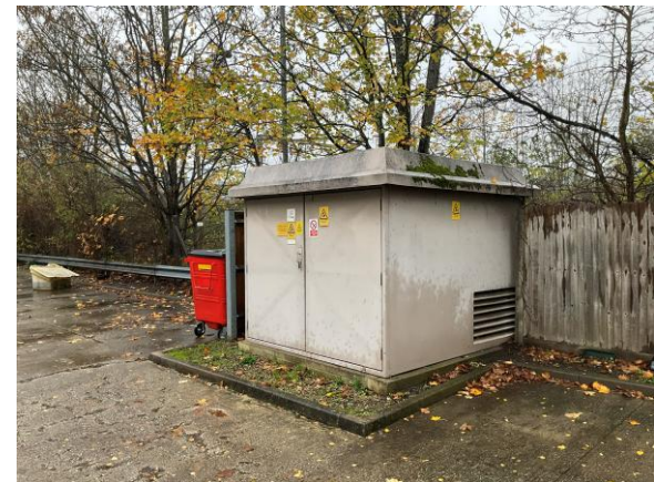
B6: Second electrical substation in north of the Site
