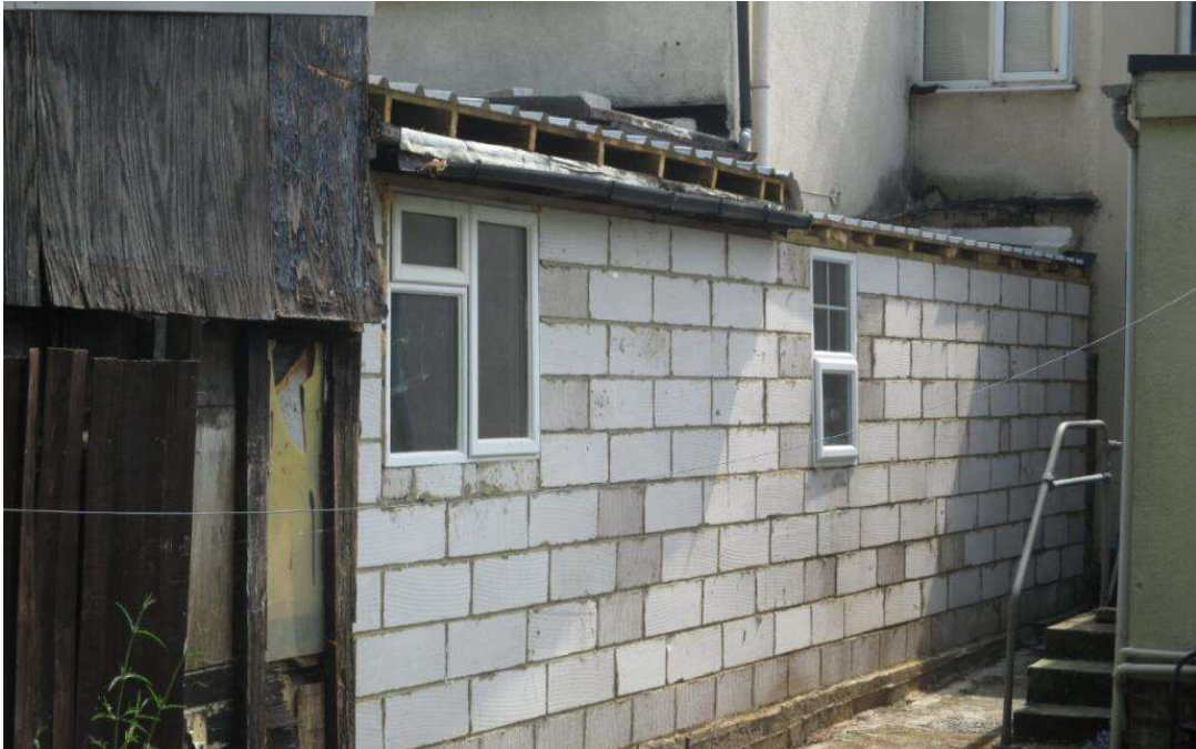
Looking towards part of the westerly facing (unauthorised) elevation overlooking the garden of no.128 Great Knollys Street.
