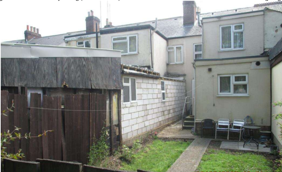
Wider photo for context; Photo shows unauthorised structure on the boundary and overlooking neighbour's outdoor amenity space.
