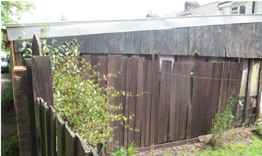
Looking towards part of the westerly facing (unauthorised) elevation constructed from timber.
