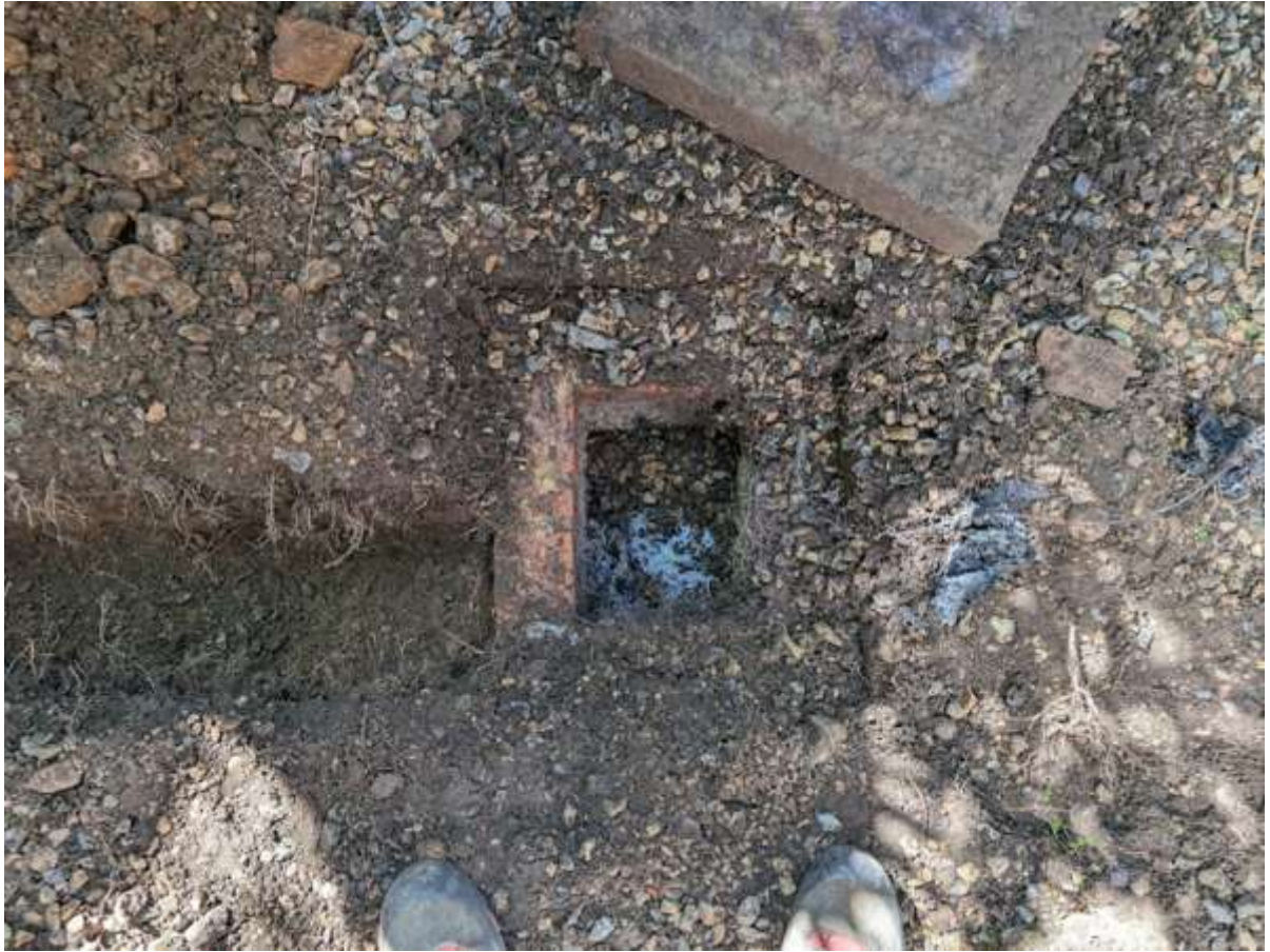
Figure 8: old drain uncovered near edge of RPA
