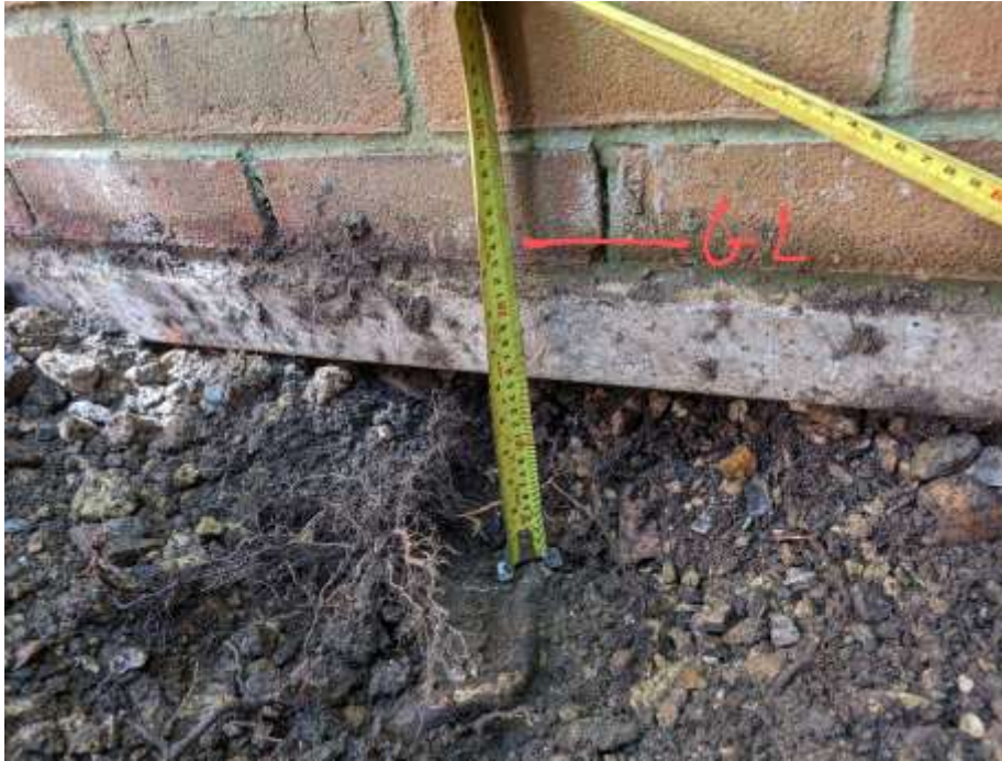
Figure 4: showing depth of root 240mm below ground level (GL)
