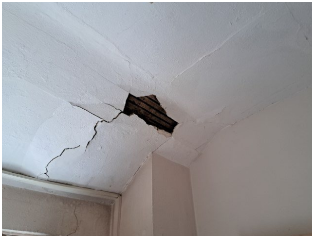
Photo 18 – View of damage in ceiling on first floor
