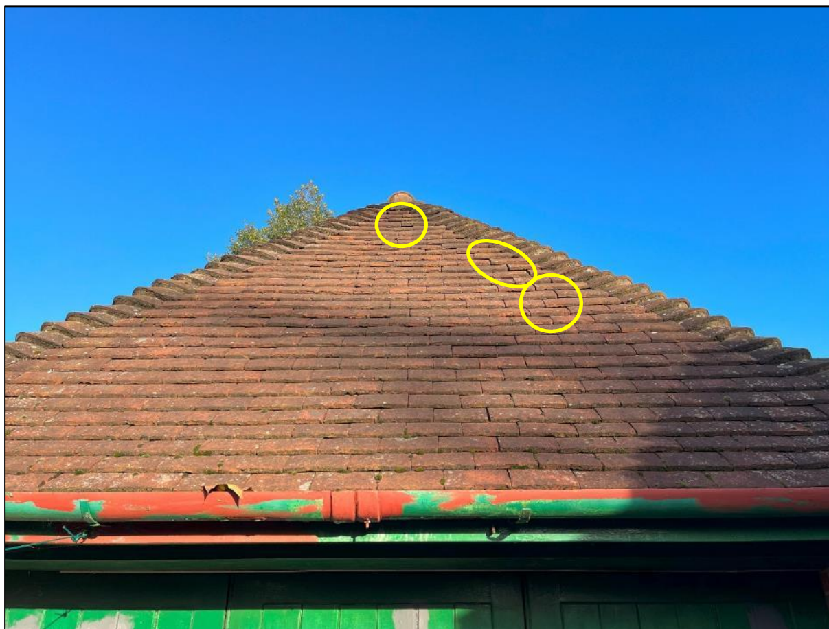
Plate 20. Gaps in the roof tiles on the western aspect of the Brick Garage.
