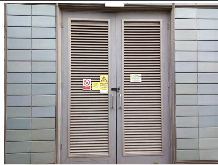
Photo 10: Electrical substation operated by SSE
