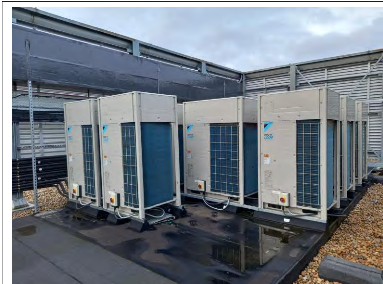
Photo 3: Air conditioning units at roof level
