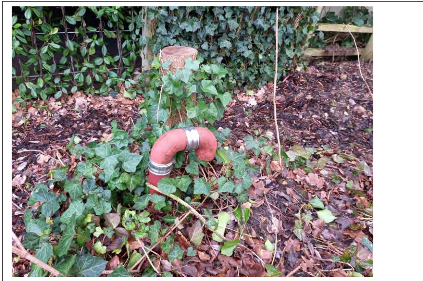
Photo 8: Associated vent pipe for interceptor (two in total)
