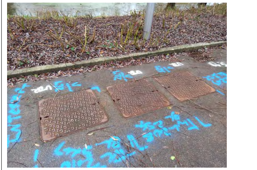
Photo 6: One of the interceptors in car park
