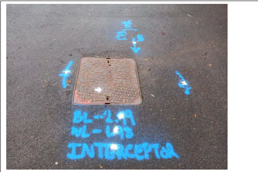
Photo 7: Second interceptor in the car park
