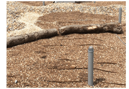
Example of air vent to brown roof
