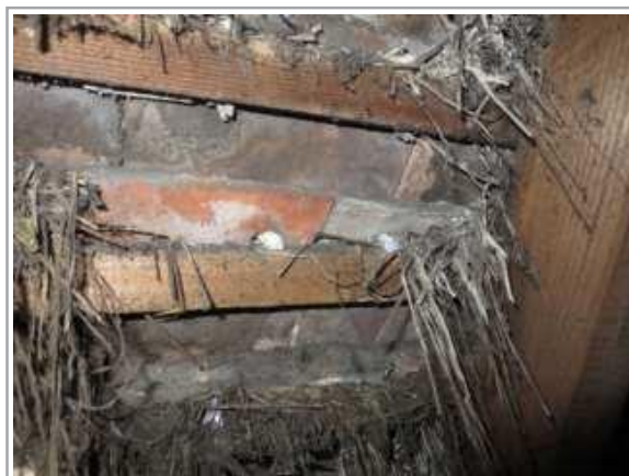
Poor tile condition
