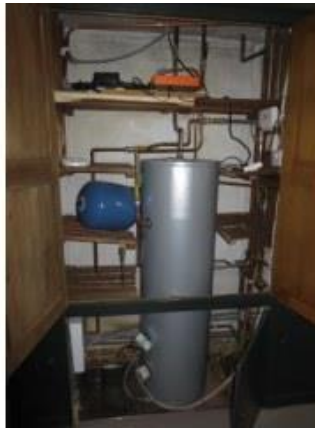
Hot water tank
