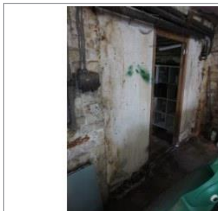
Decay garage wall
