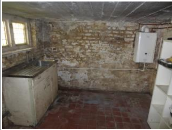
Gas boiler utility
