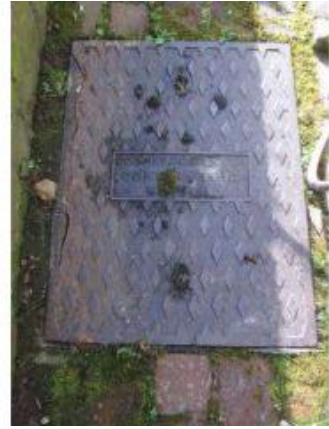
Broken drain cover.
