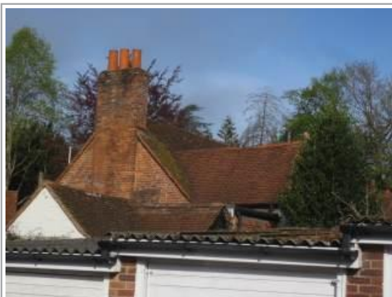
Right side stack
