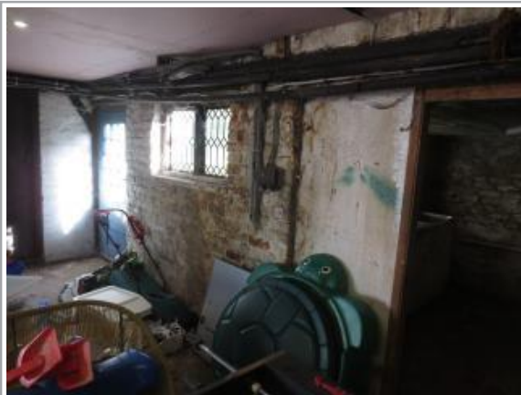
Poor pipe support.
