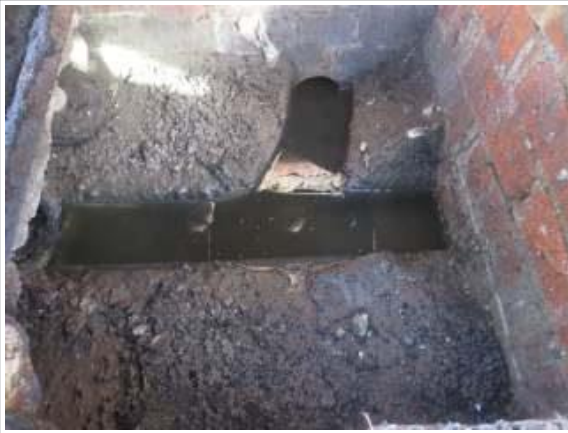
Blocked front drain.
