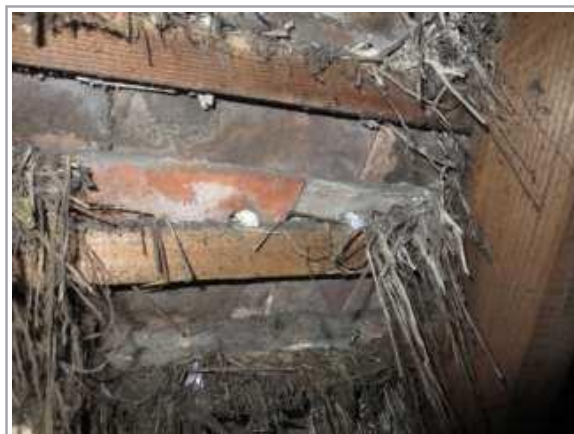
Poor tile condition
