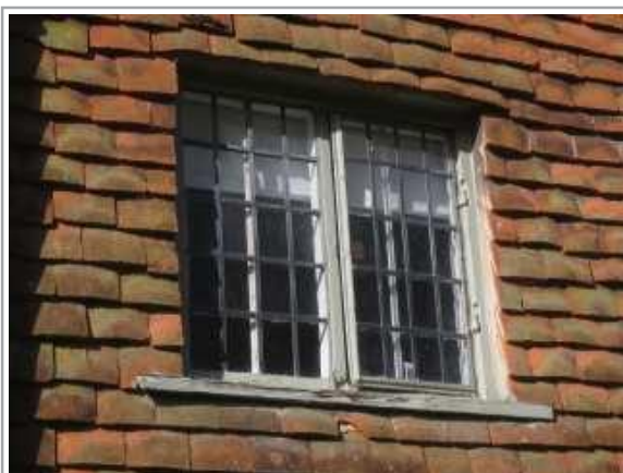
Poor window joinery
