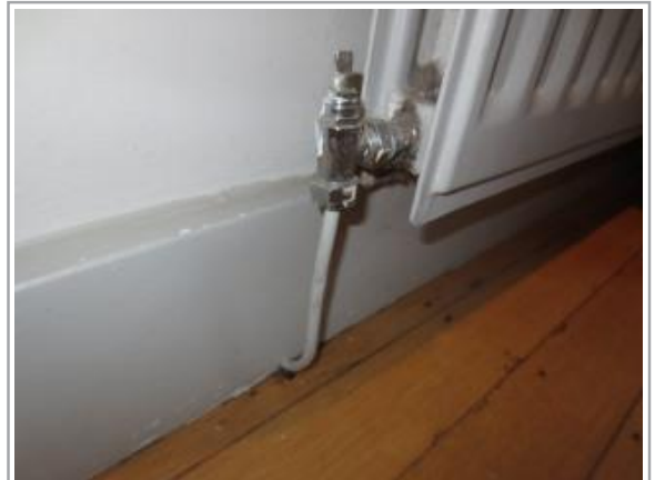
Micro bore pipes
