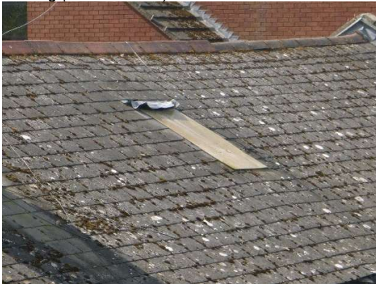
Photograph 12. Lifted lead flashing above plastic rooflight (front elevation).
