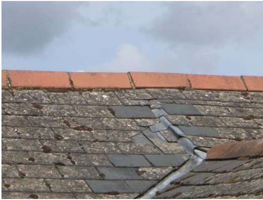
Photograph 10. Gaps beneath ridge tiles and lead flashing (rear elevation).
