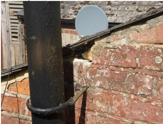
Photograph 9. Gap in verge mortar behind fluepipe (rear elevation)
