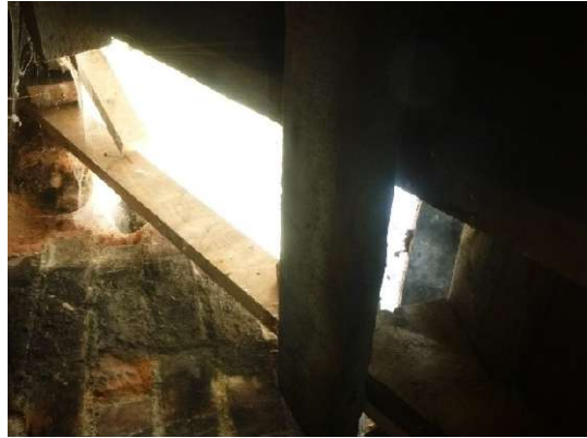
Photograph 15. Missing bitumen felting and plastic rooflight (loft space).
