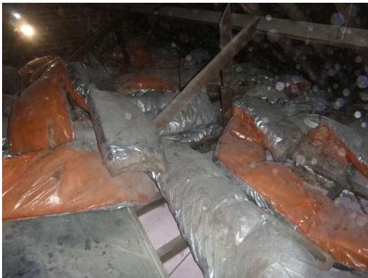
Photograph 18. Bagged fibreglass insulation (loft space).
