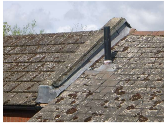
Photograph 11. Gap beneath lifted lead flashing (rear elevation).
