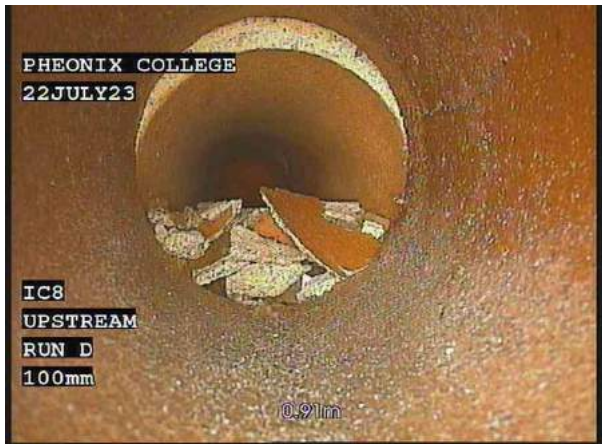
1, 00:00:25, 0.91 m Settled deposits, hard or compacted at joint, 20% cross-sectional area loss
