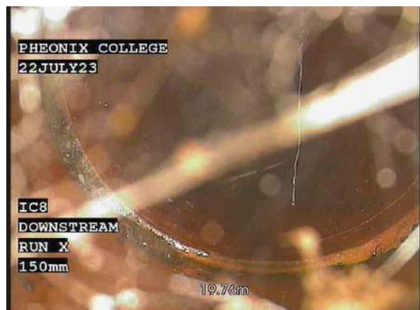
4, 00:03:11, 19.76 m Crack, circumferential at joint from 04 o'clock to 05 o'clock
