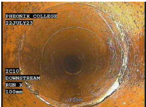
1, 00:00:08, 0.55 m Crack, circumferential from 09 o'clock to 02 o'clock
