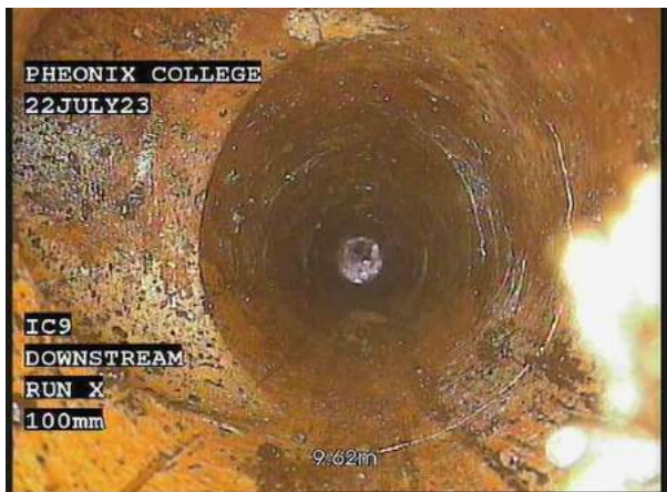
3, 00:01:23, 9.62 m Crack, circumferential from 02 o'clock to 06 o'clock
