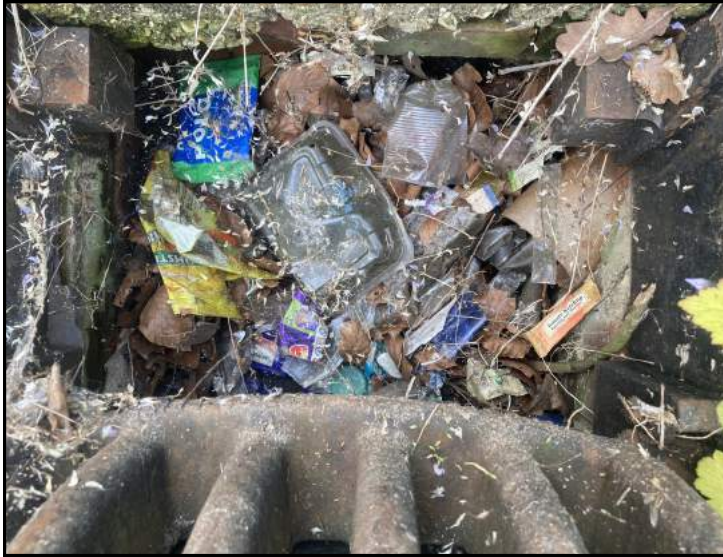
GULLY 1 - DEBRIS FILLED
