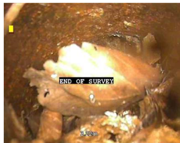
4, 00:00:28, 3.22 m Survey abandoned, Unable to continue due to debris
