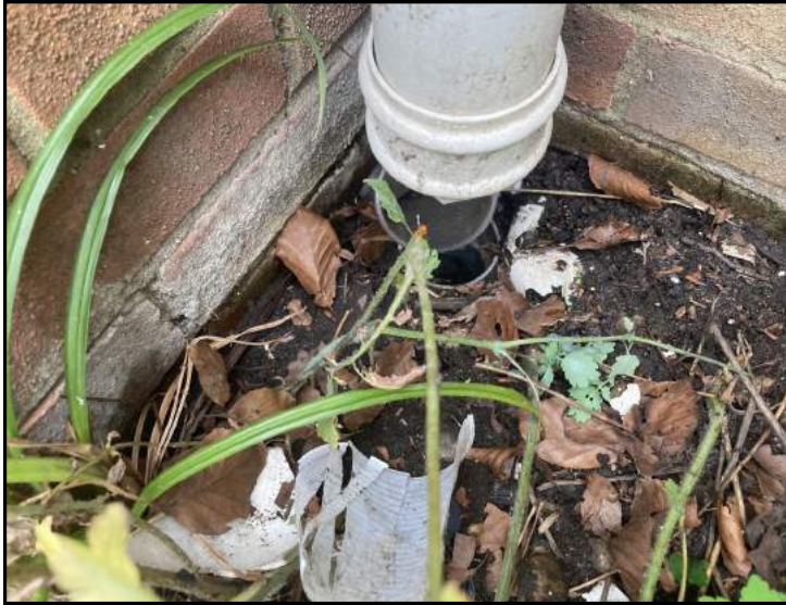
RWP 6. 65mm PVC OUTFALL. UNABLE TO CCTV
