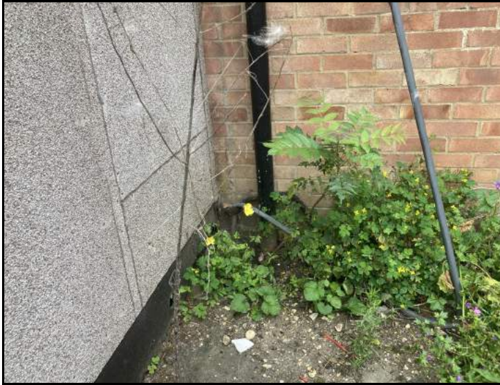
RWP 3 - APPEARS TO BE UNCONNECTED
