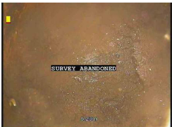
3, 00:01:37, 6.23 m Survey abandoned, Unable to pass due to silt deposits
