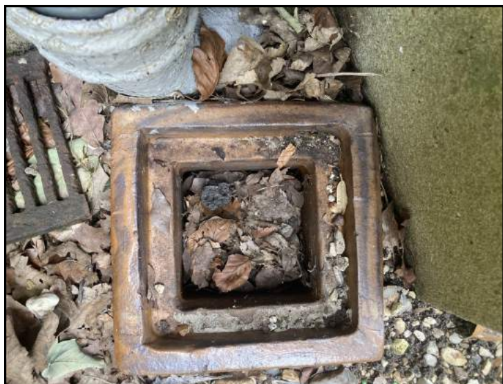
GULLY 7 - DEBRIS FILLED
