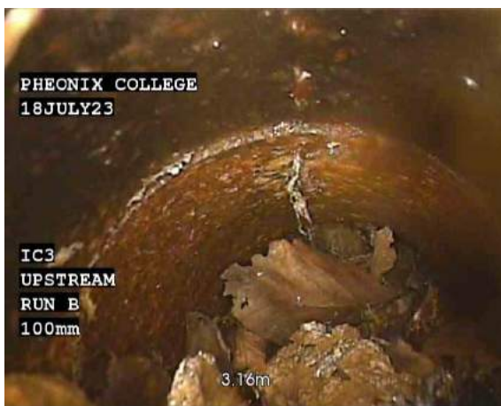
3, 00:00:22, 3.16 m Settled deposits, hard or compacted, 80% cross-sectional area loss
