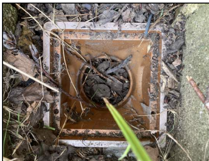
RWP 2 - DEBRIS FILLED
