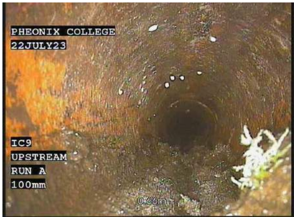
1, 00:00:08, 0.66 m Settled deposits, hard or compacted, 5% cross-sectional area loss, start
