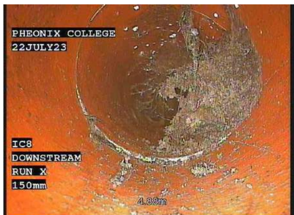
1, 00:00:26, 4.88 m Roots, mass at joint, 25% cross-sectional area loss
