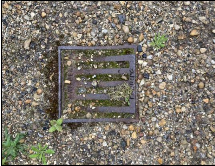
GULLY 4 - DEBRIS FILLED
