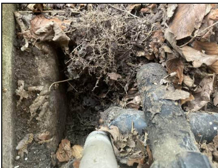
GULLY 6 - DEBRIS FILLED
