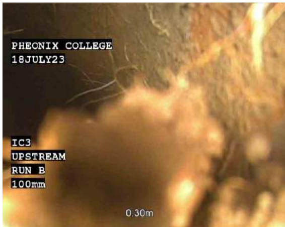
1, 00:00:01, 0.30 m Settled deposits, hard or compacted, 15% cross-sectional area loss, start
