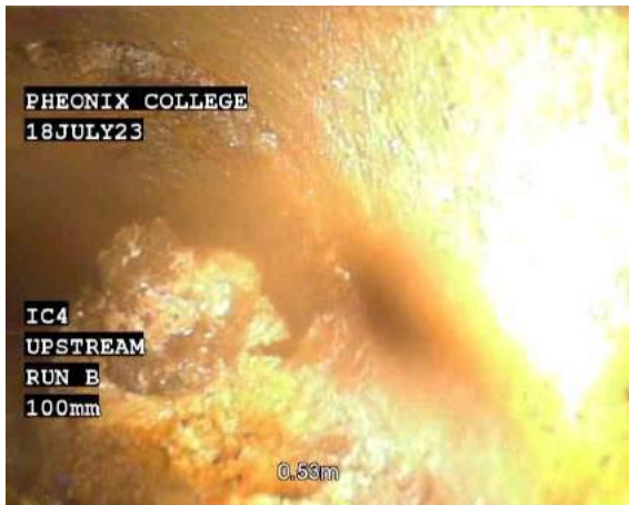
1, 00:00:07, 0.53 m Settled deposits, hard or compacted, 50% cross-sectional area loss, start
