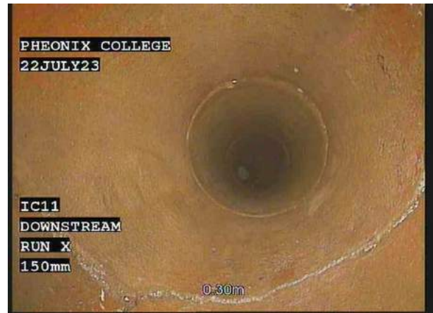
2, 00:00:24, 0.30 m Fracture, circumferential at joint from 03 o'clock to 09 o'clock
