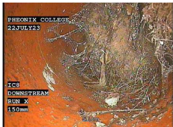
2, 00:00:41, 5.16 m Roots, mass, 80% cross-sectional area loss
