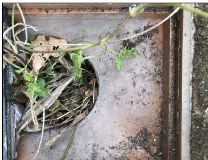
RWP 1 - DEBRIS FILLED
