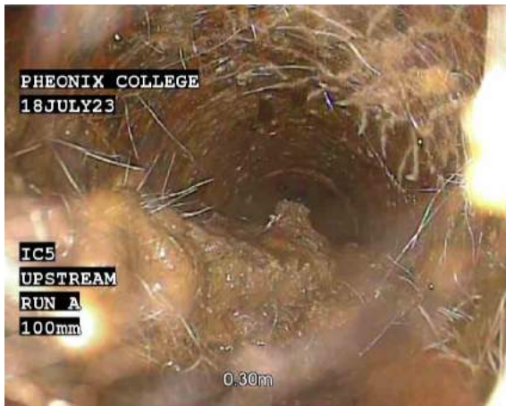
1, 00:00:00, 0.30 m Settled deposits, hard or compacted, 30% cross-sectional area loss, start
