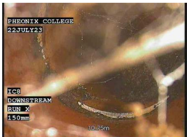
3, 00:02:12, 10.75 m Settled deposits, hard or compacted at joint, 20% cross-sectional area loss
