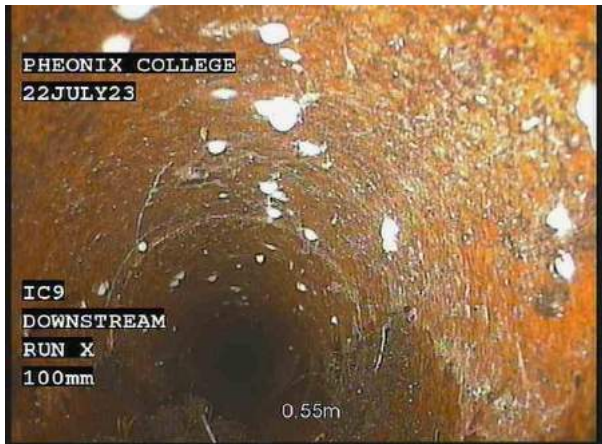
1, 00:00:10, 0.55 m Settled deposits, hard or compacted, 5% cross-sectional area loss, start
