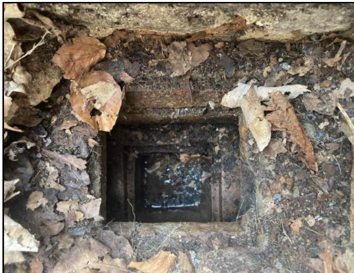
GULLY 5. TRAPPED - NO CCTV
