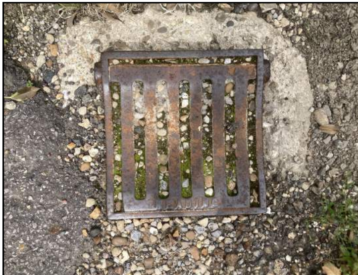
GULLY 2 - DEBRIS FILLED
