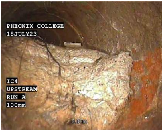
1, 00:00:00, 0.00 m Settled deposits, hard or compacted, 60% cross-sectional area loss, start
