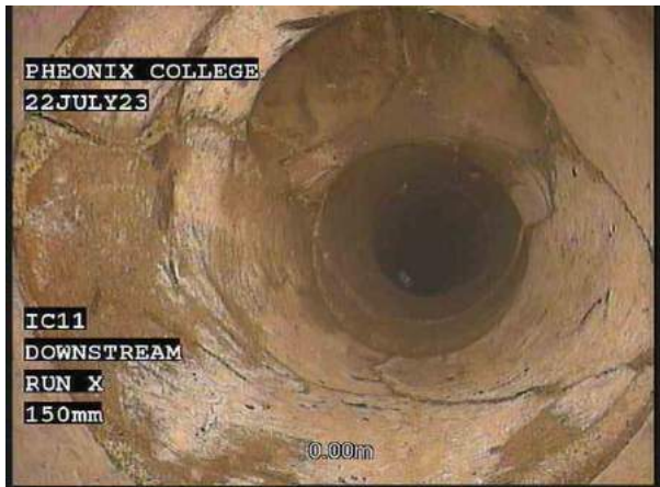
1, 00:00:04, 0.00 m Fractures, multiple from 12 o'clock to 12 o'clock
