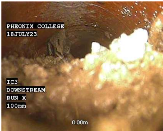
1, 00:00:00, 0.00 m Settled deposits, hard or compacted, 50% cross-sectional area loss, start
