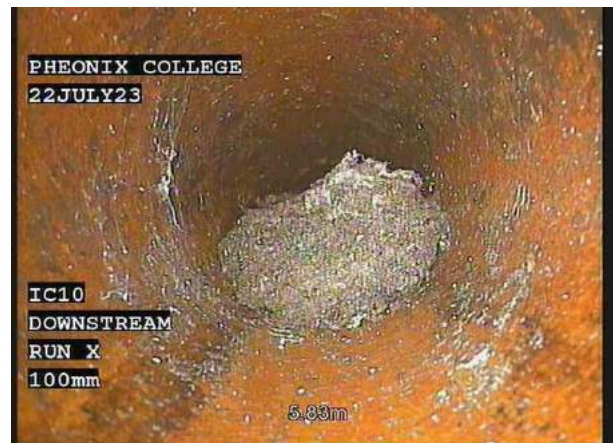
2, 00:00:45, 5.83 m Settled deposits, hard or compacted, 50% cross-sectional area loss
