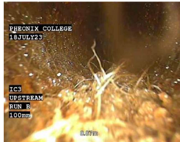
2, 00:00:10, 0.87 m Settled deposits, hard or compacted, 5% cross-sectional area loss, start
