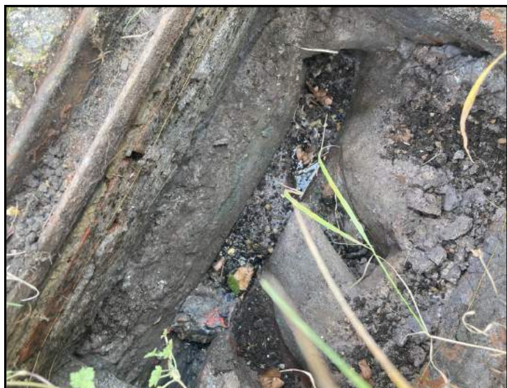
IC4. MANHOLE SILTED
