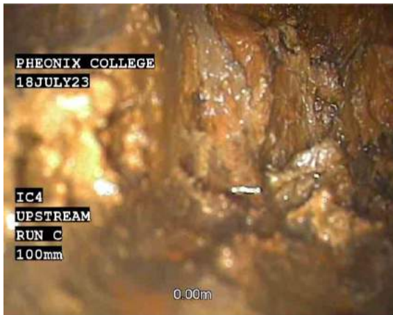
1, 00:00:01, 0.00 m Settled deposits, hard or compacted, 60% cross-sectional area loss, start
