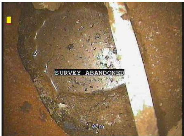
3, 00:01:18, 1.97 m Survey abandoned, Unable to continue - assumed debris filled interceptor / trap
