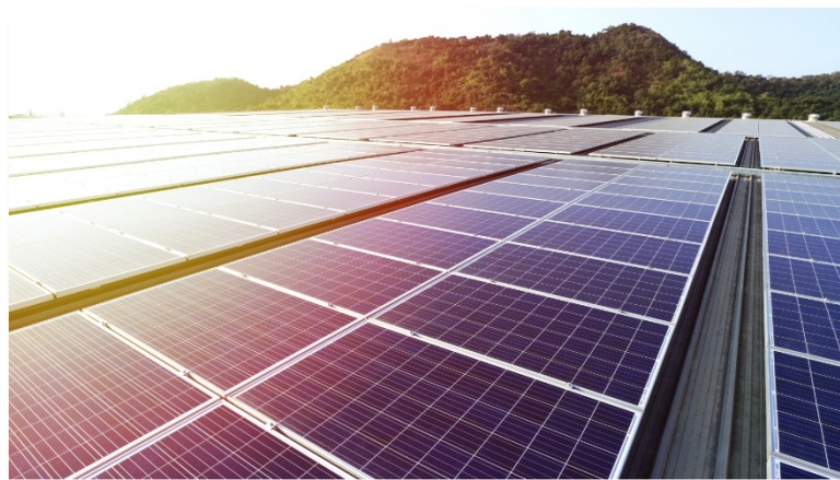
Typical Roof Mounted PV Array
