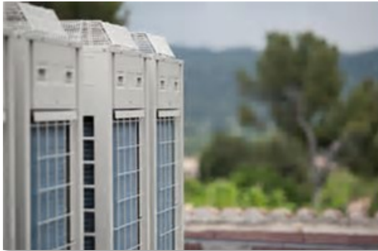
Typical ASHP Outdoor Units
