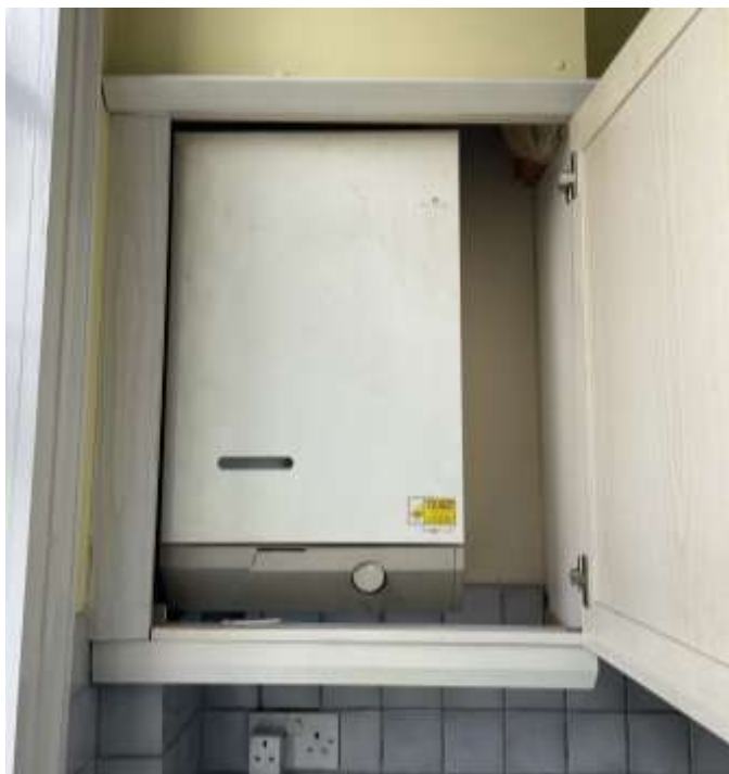
Existing boiler in kitchen
