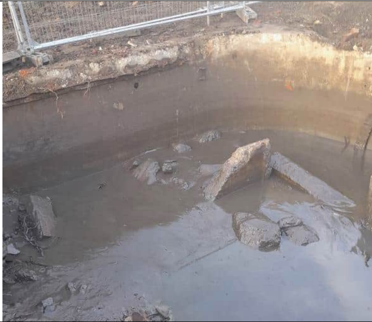
Photograph 1: Collection of waste water on site.
