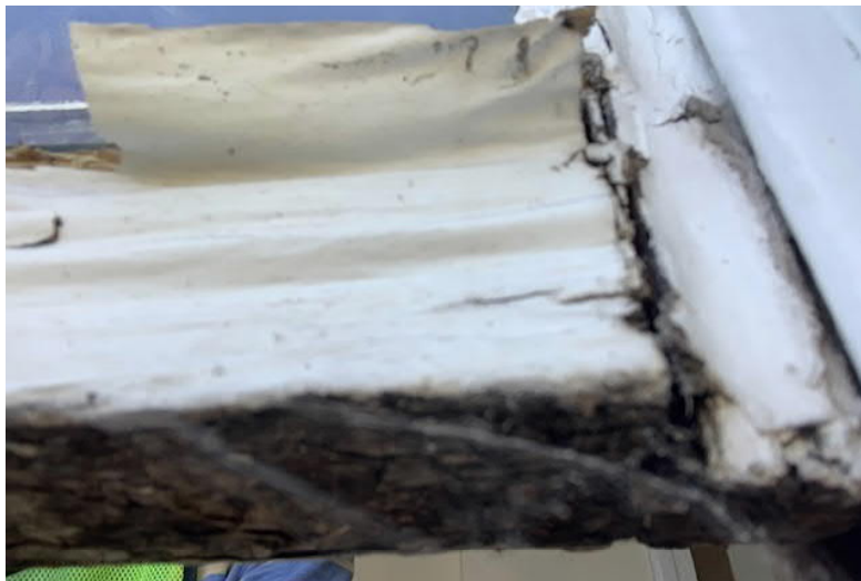
Image 34b: View of bottom rail of sliding sash of central sash window - the joint has opened and caused the timber to rot
