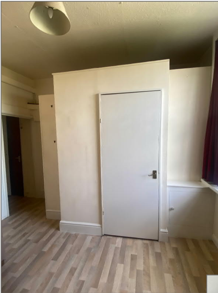
Image 30: Bathroom enclosure, Flat 5
