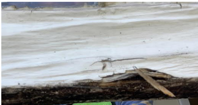
Image 34c: View of bottom rail of sliding sash of central sash window - the paint has failed and the timber below appears to be rotting
