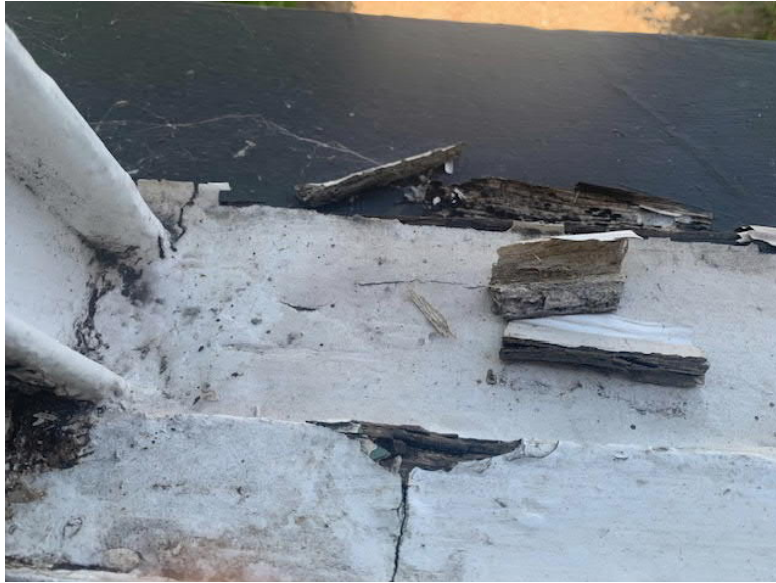
Image 34a: View of timber cill of central sash window - the paint has cracked open and water has become trapped beneath it causing the timber to rot
