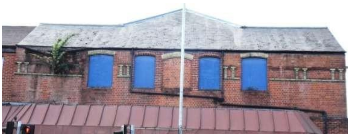
Fig 3.3.12: Upper section of Caversham Road front to N° 73
