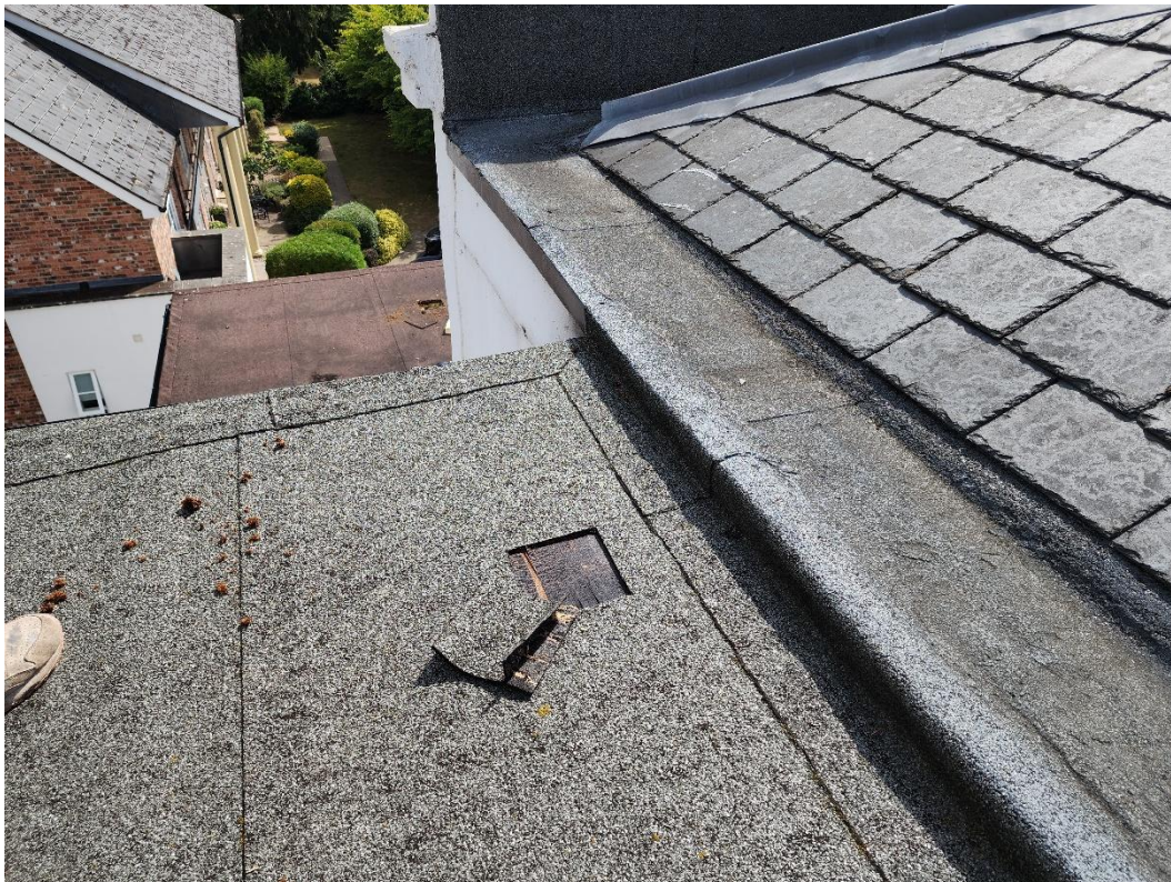
Photo 15 – Core sample 5 (Upper section of roof area 4) – Felt directly onto plywood.
