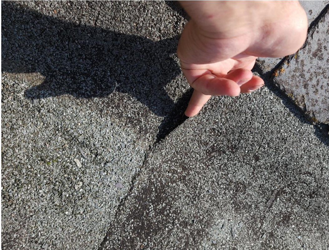
Photo 8 - Poorly bonded joint to roof 3.
