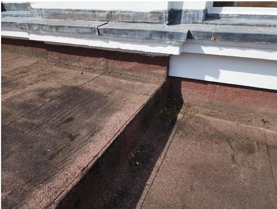
Roof 1 (upper) and Roof 2 (Lower) – note 'ruckled' felt)
