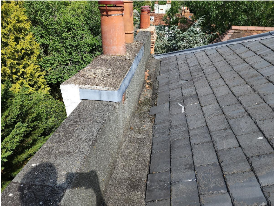
Photo 10 – Opposite side of roof 3 parapet detail. Note slipped and cracked slates.
