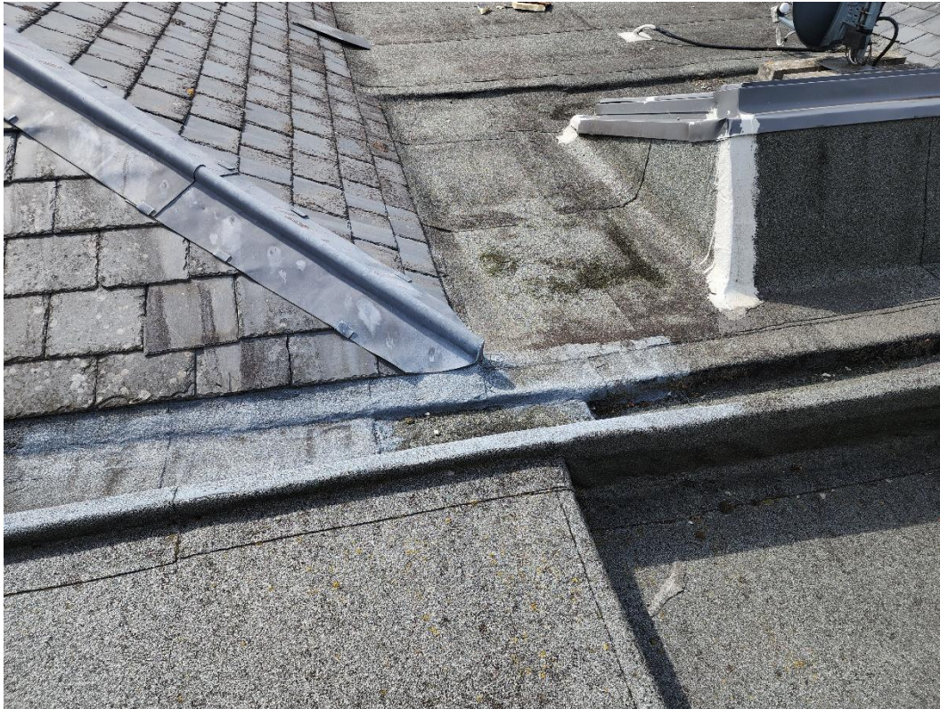
Photo 14 - Unnecessary detailing to step between Roof 3 and Roof 4. Note liquid applied coating.
