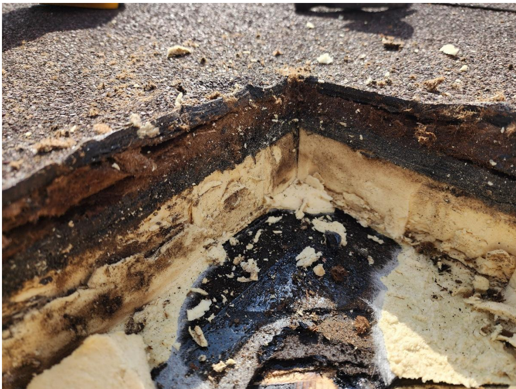
Photo 2 - Core 2 – Note damp fibre board over insulation.
