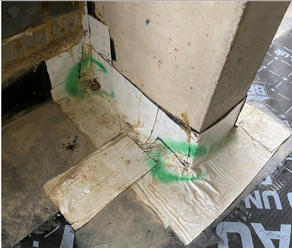
Photograph 9: Areas sprayed from previous Hydrock visit not rectified.
