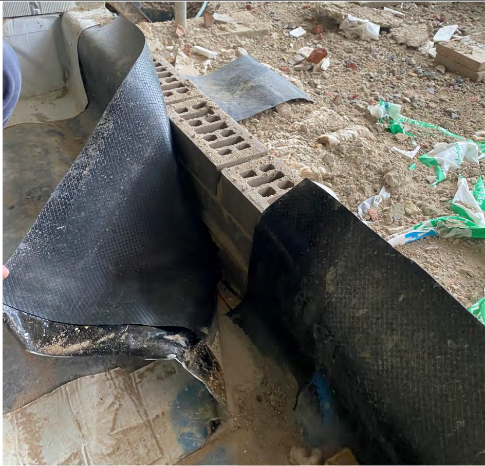
Photograph 11: Membrane not sealed and has come away from brickwork
