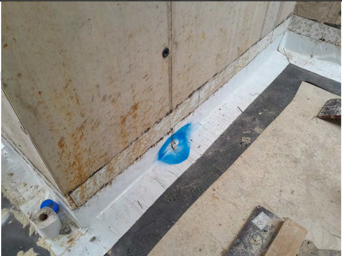
Photograph 12: possible defect in detail tape joint
