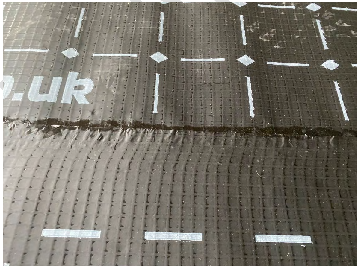
Photograph 4: Seals noted with &lt;100mm overlapping.
