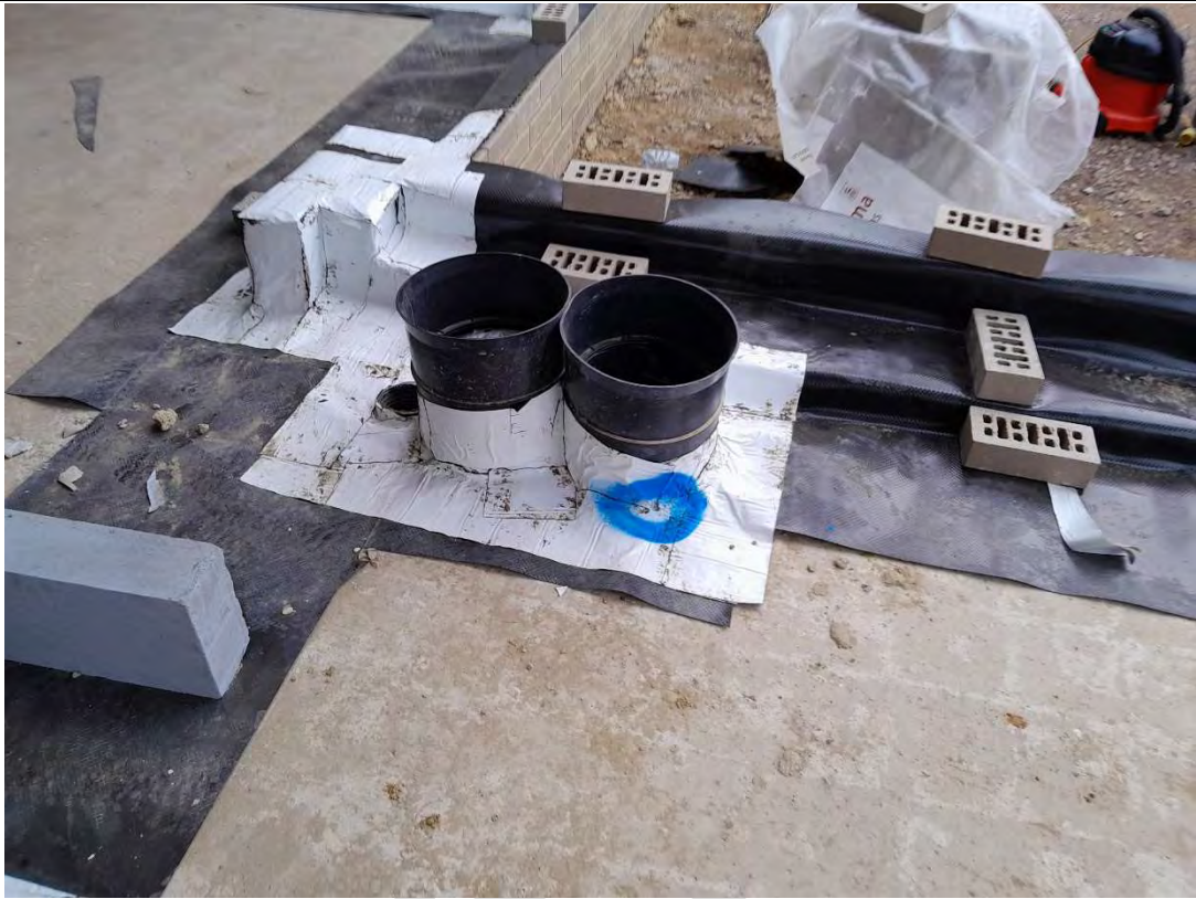
Photograph 11: possible defect in service entrance seal
