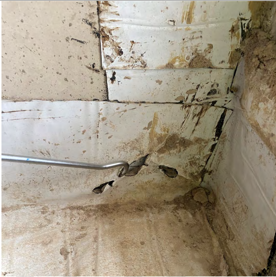
Photograph 7: Damage noted on lapping joints/seals.
