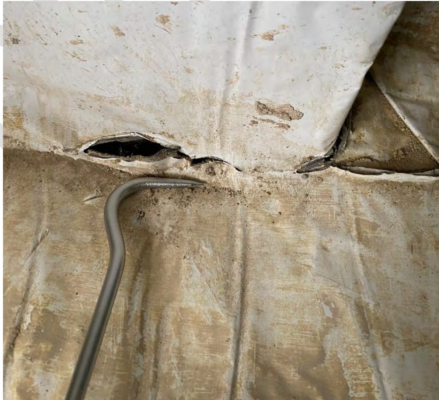
Photograph 8: Damage noted on lapping joints/seals.
