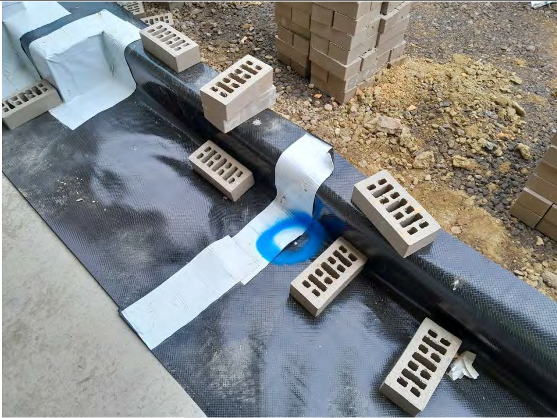
Photograph 9: possible defect in join lapping seal
