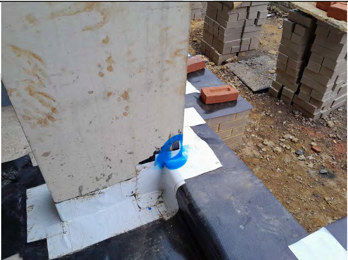
Photograph 10: possible defect in adhesion to pillar
