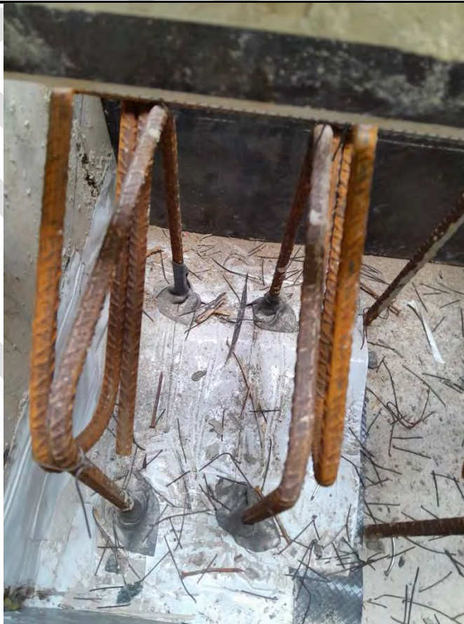
Photograph 8: Detailing around reinforcement bar penetrating DPC
