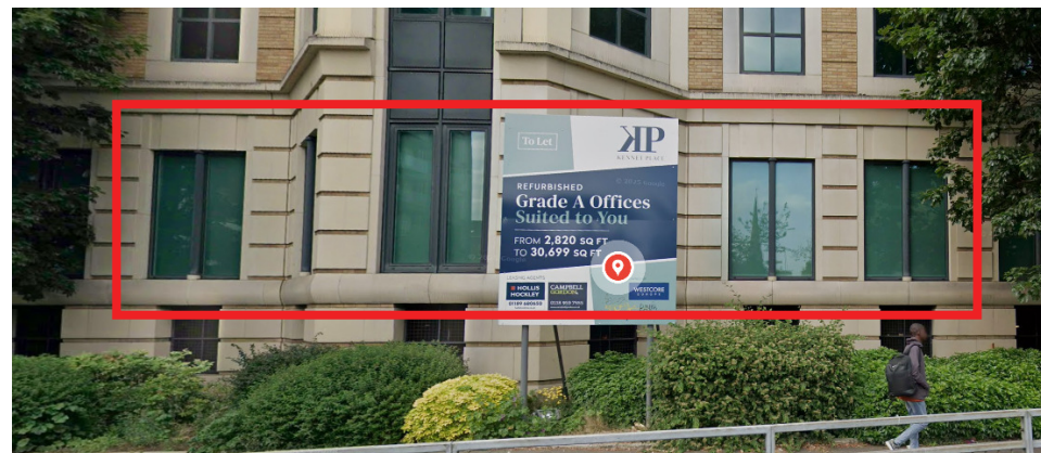
Example of existing fixed windows on the Kings Road Elevation at 'Ground Floor' which once replaced with an openable function would present a fall risk to the occupants.
