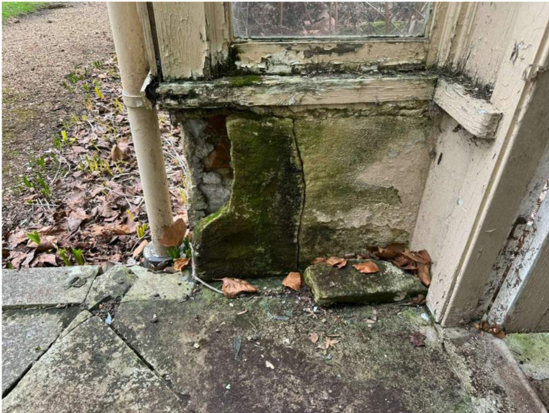
Photograph 34 – Damp and fractured render to plinth wall.
