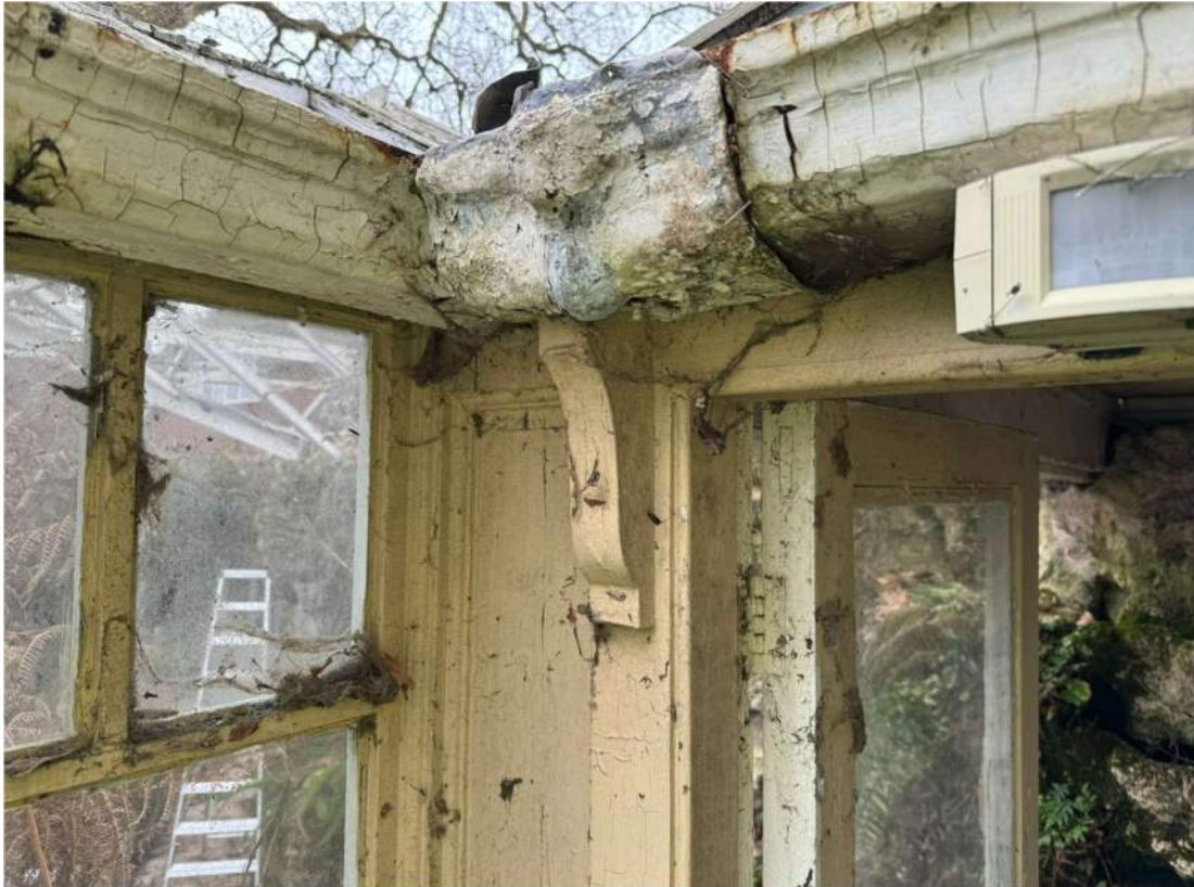
Photograph 37 – Perished cast iron gutters.
