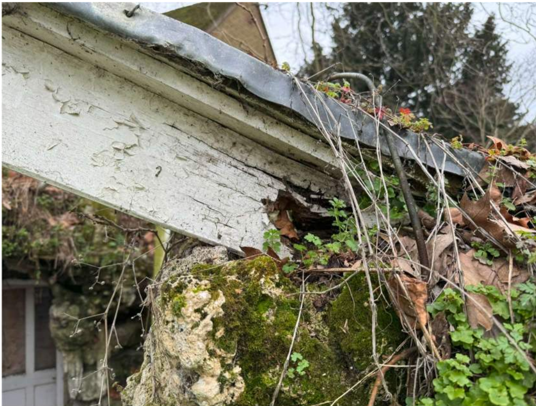
Photograph 10 – Severe decay at end of principal rafter
