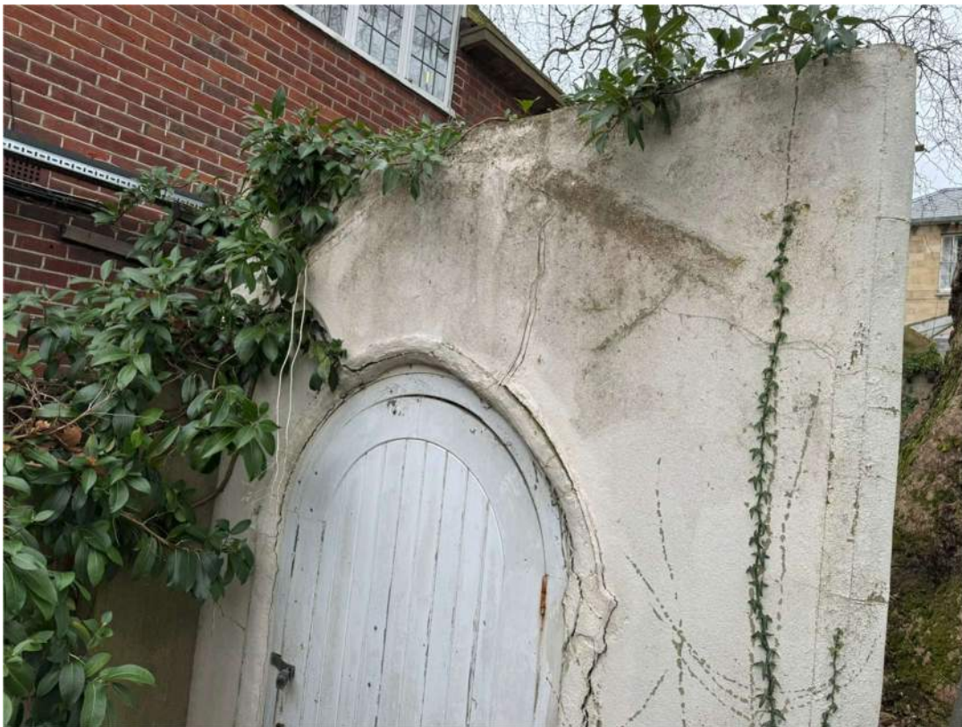
Photograph 46 – Historic and repaired cracking above entrance arch.
