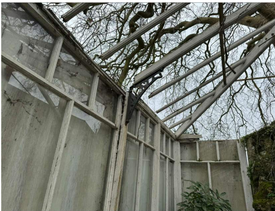
Photograph 20 – Several decayed ends to principal rafters and decayed glazing bars
