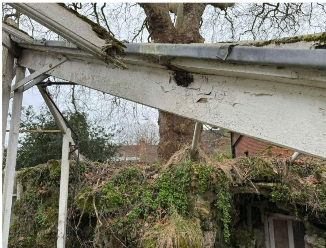
Photograph 11 – Severe decay to glazing bar and loss of support.
