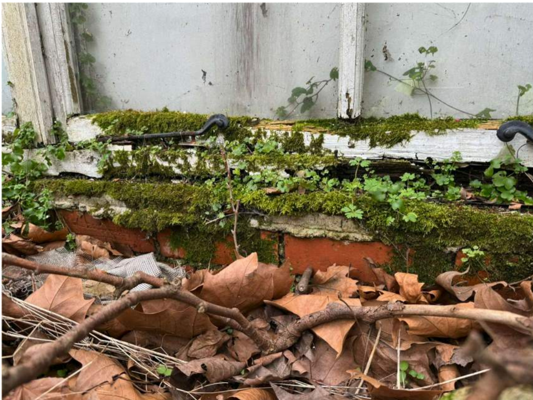
Photograph 38 – Perished timber wall plate along brick plinth wall
