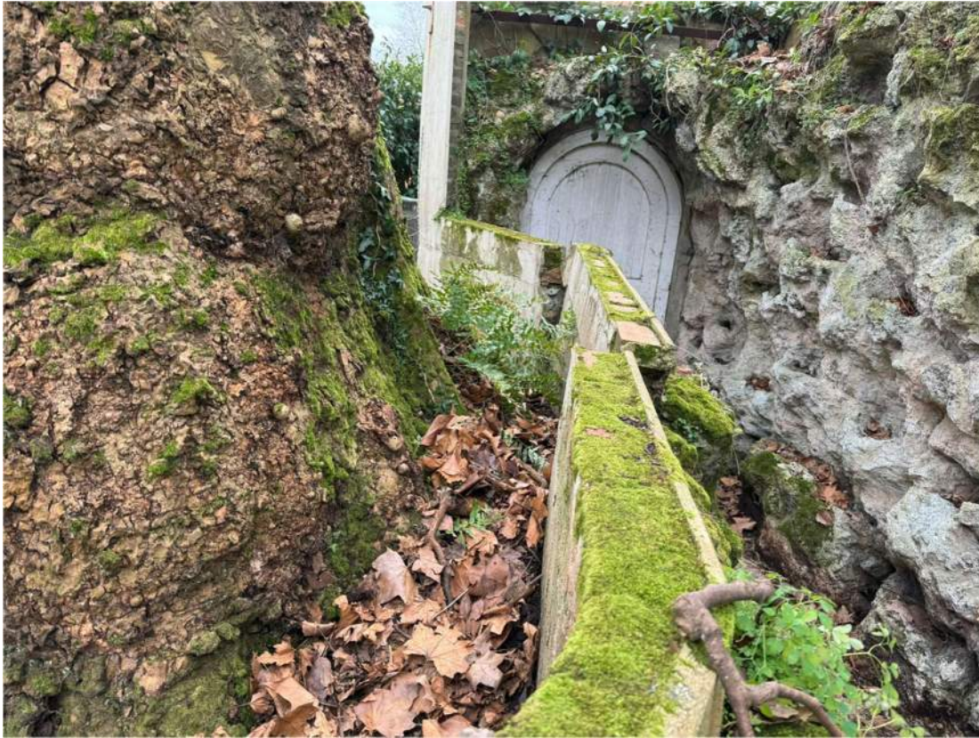
Photograph 43 – Proximity of London Plane tree and severe displacement of plinth wall.
