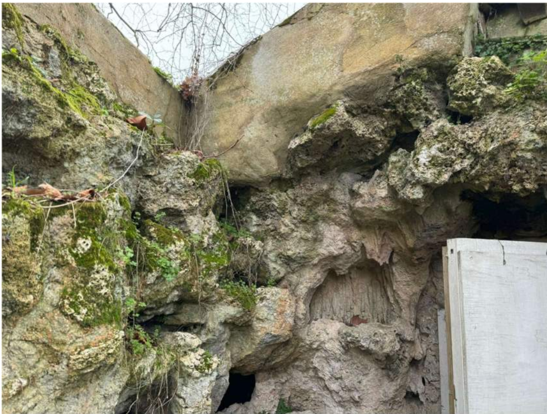
Photograph 40 – Pulhamite wall in corner of corridor and location of 5mm vertical crack
