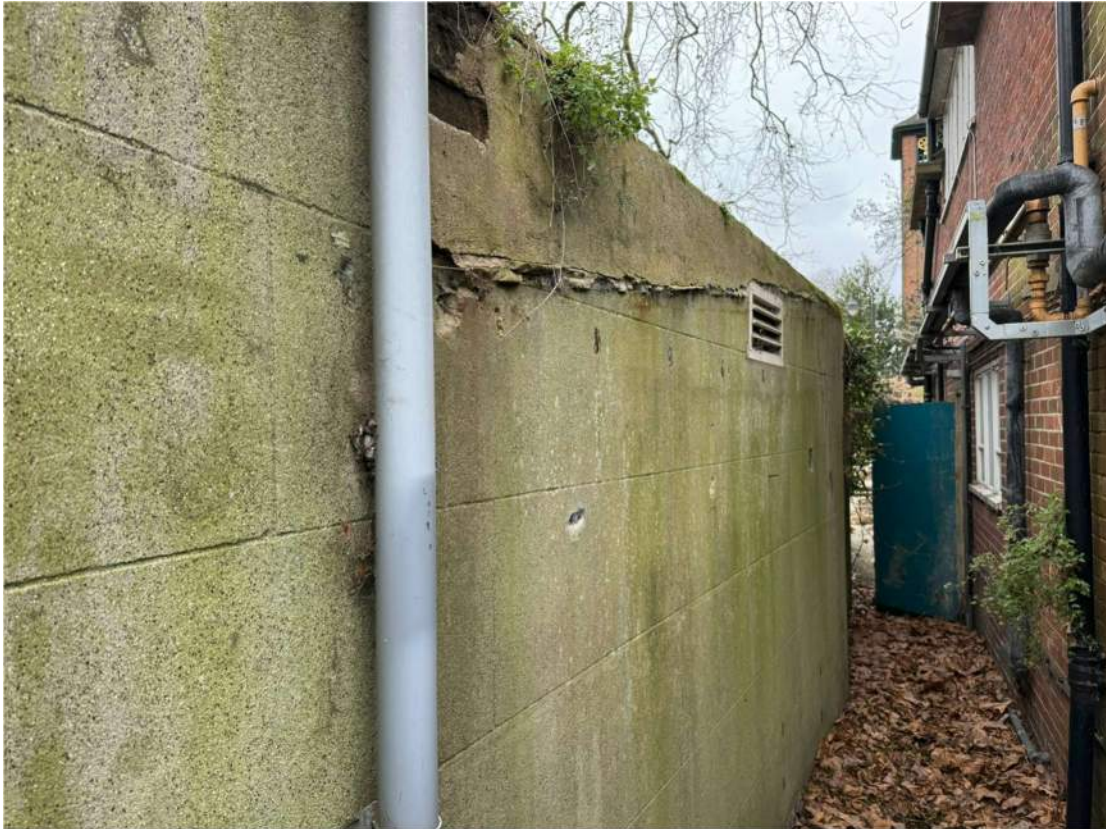
Photograph 51 – Render rear to the corridor wall and some hairline cracking.
