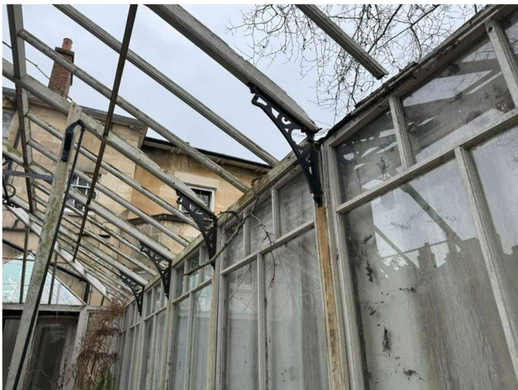
Photograph 19 – Several decayed ends to principal rafters at junction with cast iron brackets. Note glass protected by plywood.
