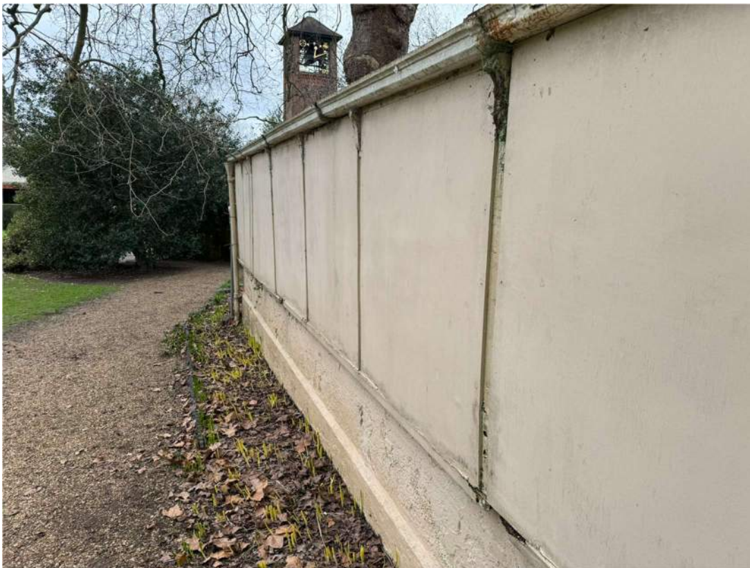
Photograph 36 – Outwards lean to timber posts and frame.
