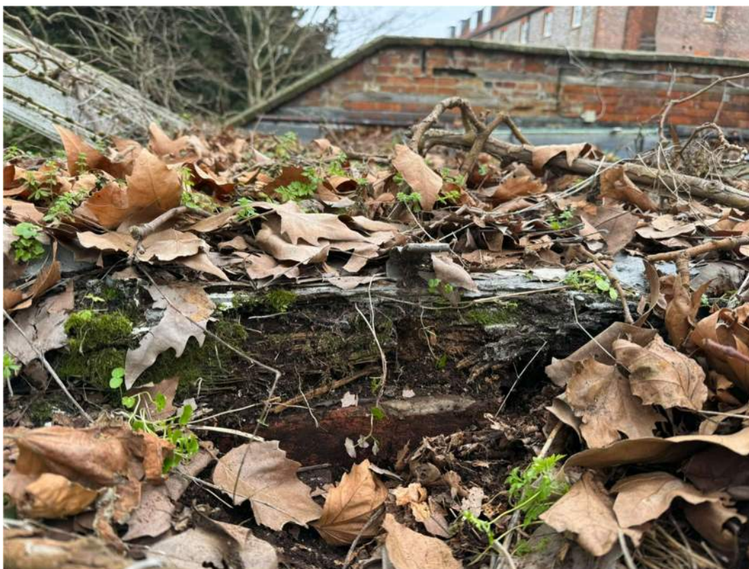
Photograph 13 – Wall plate above west wall is perished.
