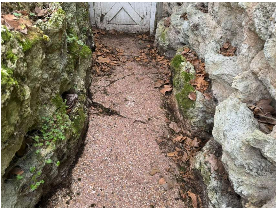
Photograph 44 – Cracking and movement in ground bearing concrete slab beside London Plane.
