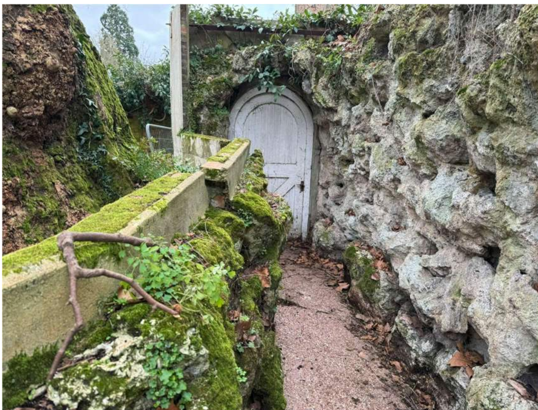
Photograph 42 – 90 – 150mm displacement in wall over 1400mm height.
