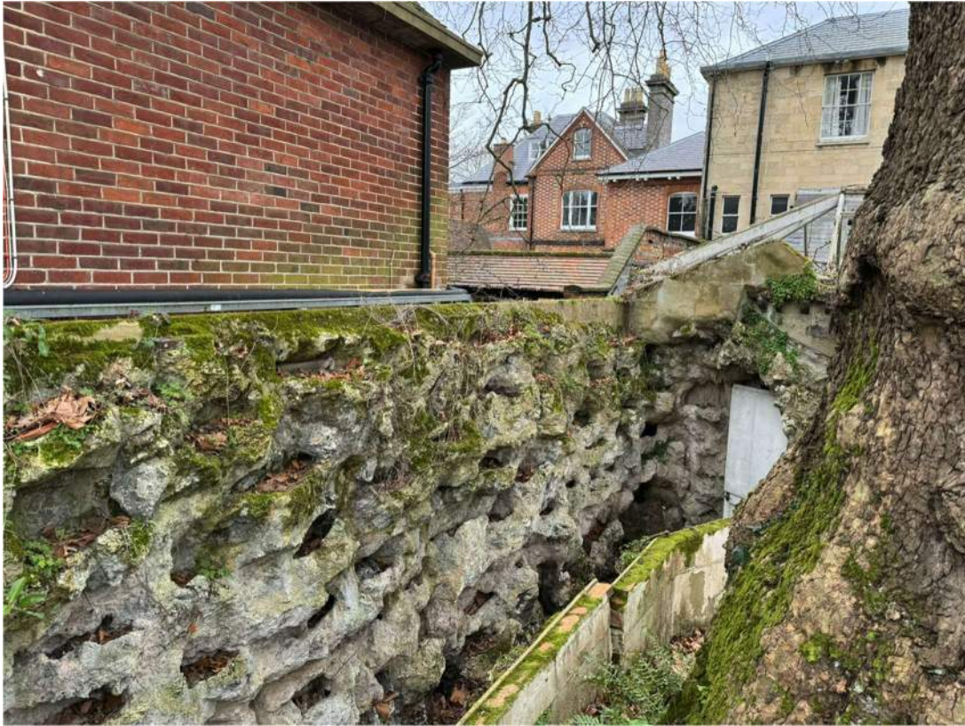
Photograph 49 – Rear corridor wall has some minor lean of around 5mm.
