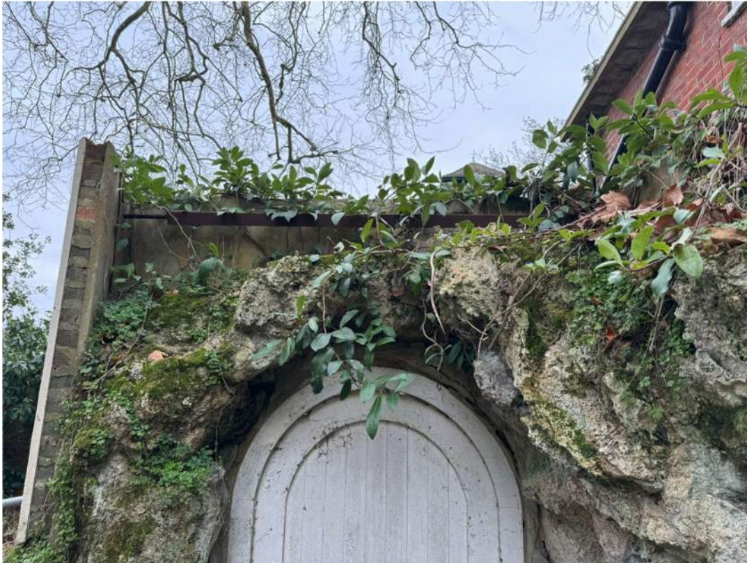
Photograph 47 – Earlier remedial tie bar above entrance arch.
