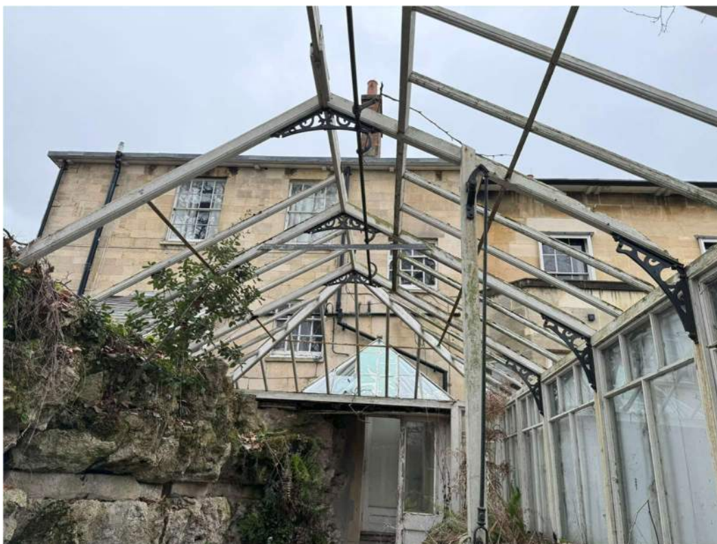
Photograph 18 – Decayed ends to principal above cast iron eaves brackets.
