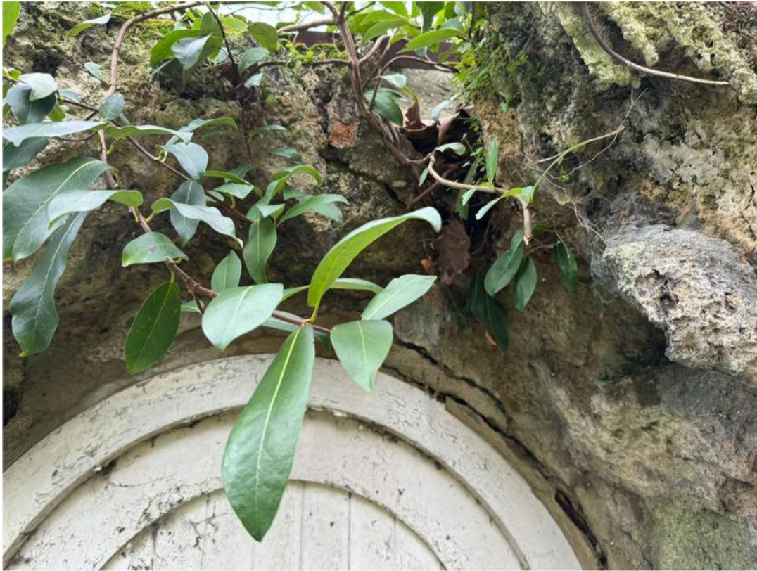
Photograph 45 – Cracking above entrance arch to corridor.
