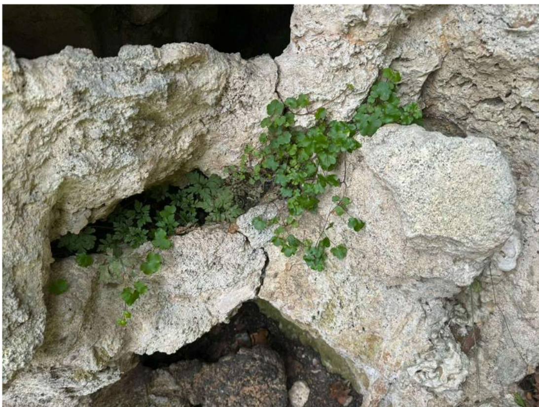
Photograph 41 – Detail of 5mm vertical crack in Pulhamite wall.
