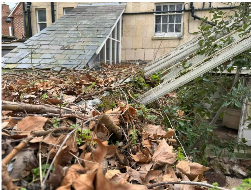
Photograph 12 – Timber wall plate above the west wall has limited access and traps water easily.
