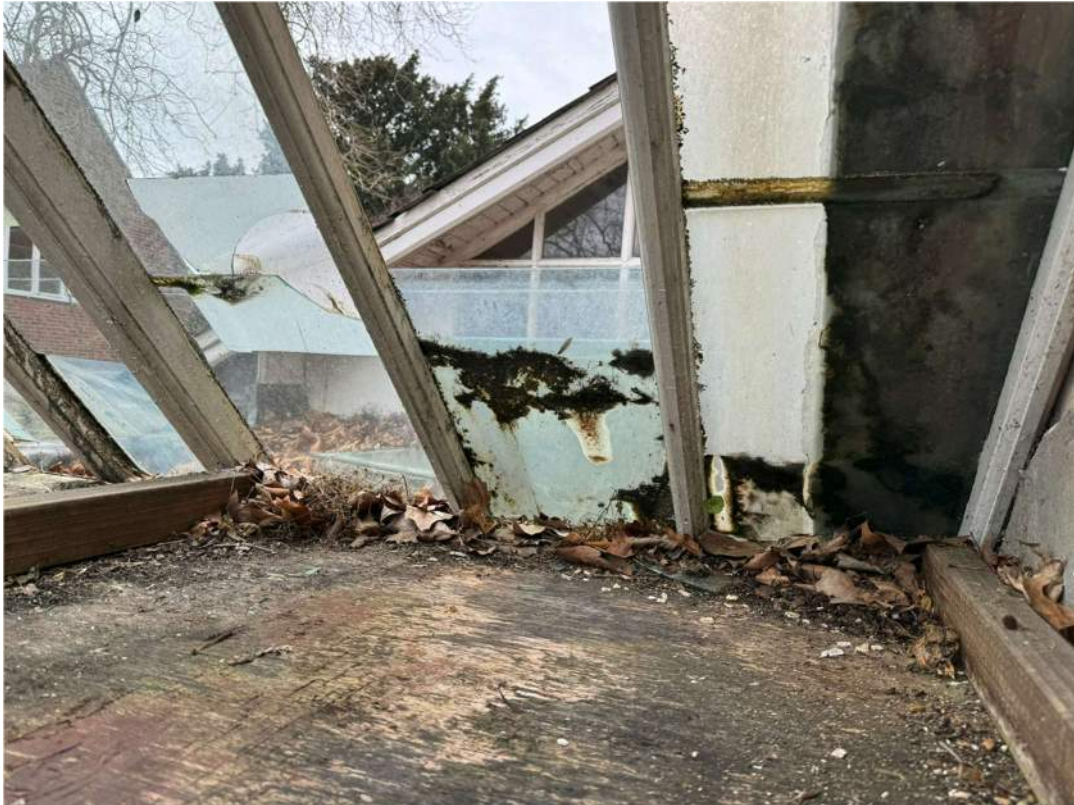
Photograph 33 – Ply crash deck with glazing and glazing bars above. Some glass panels missing.
