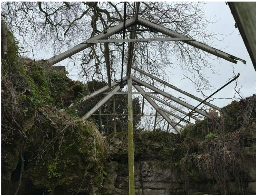
Photograph 17 - Decayed ends to principal rafters and lack of support.
