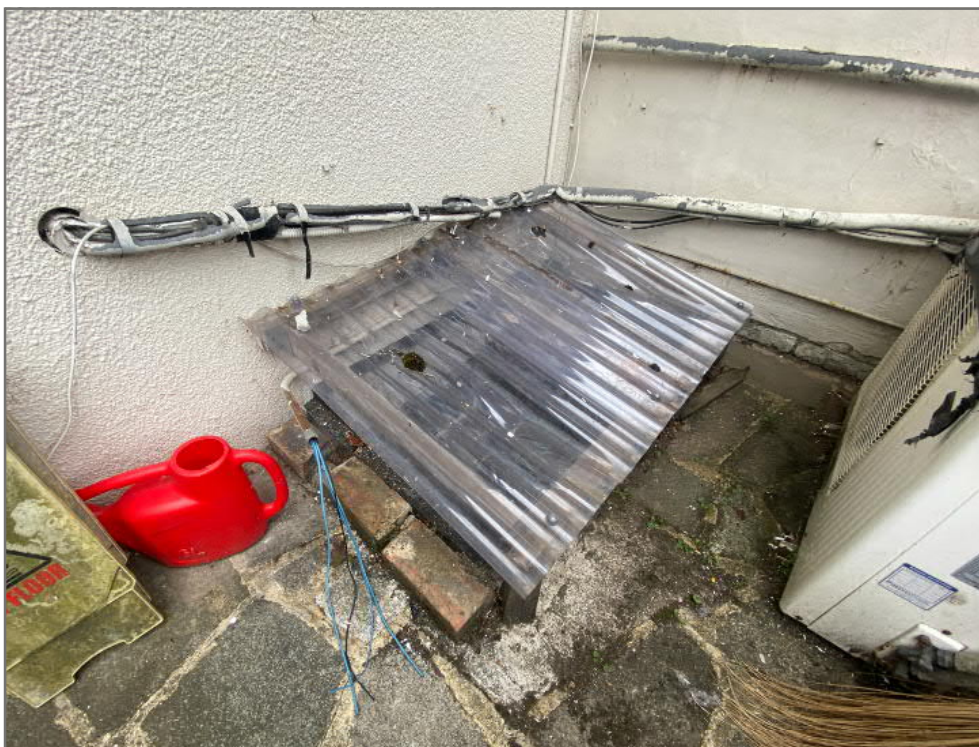
Image 32: Basement window protected from water ingress
