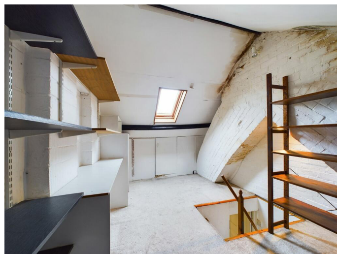
Figure 7: Existing converted loft with ladder stairs and velux window. Roof water damage to chimney surrounds also evident.
