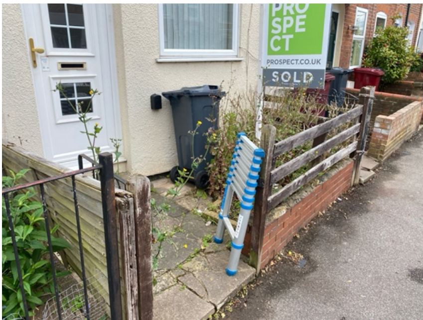
Figure 3: Existing front garden with poor condition paving, wall and railings
