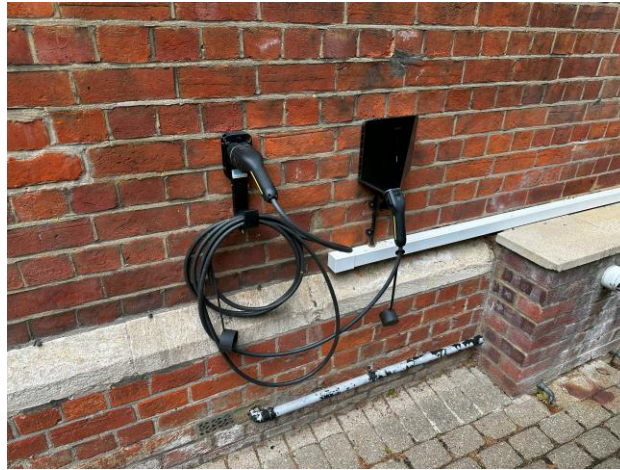
Figure 11 – Existing EV charger
