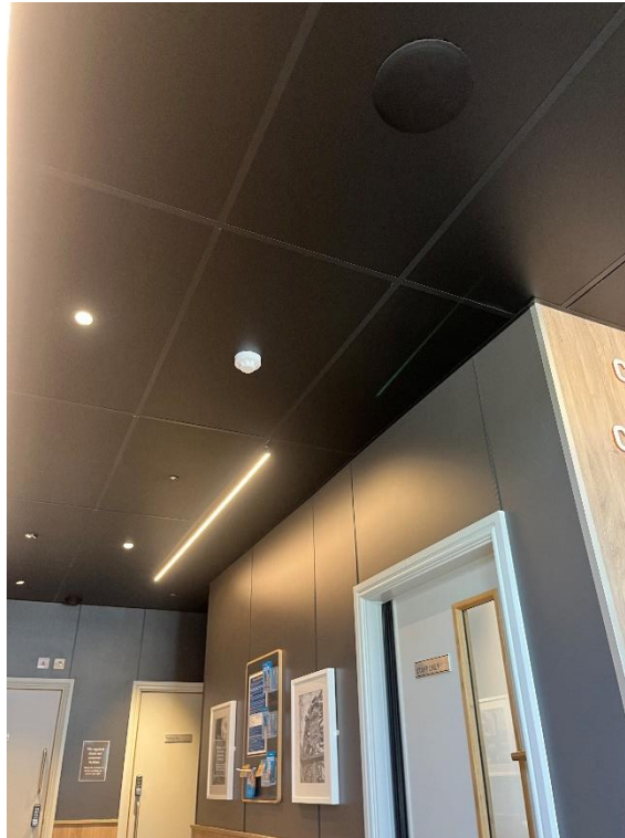
Internal Light Fittings
