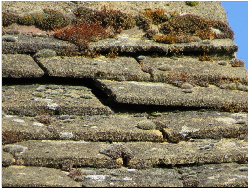
Photograph J Crevices under roof tiles, with bat roosting potential
