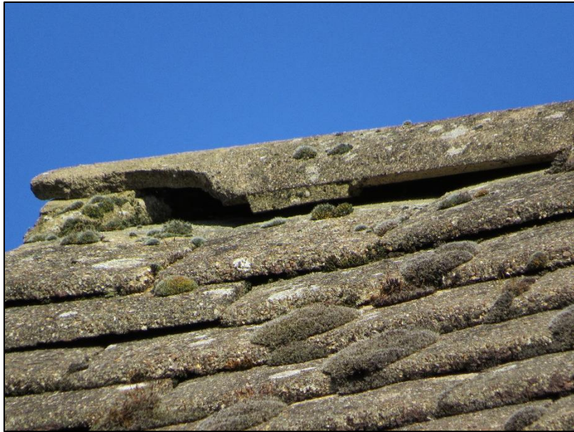
Photograph I Crevice under a ridge tile, with bat roosting potential
