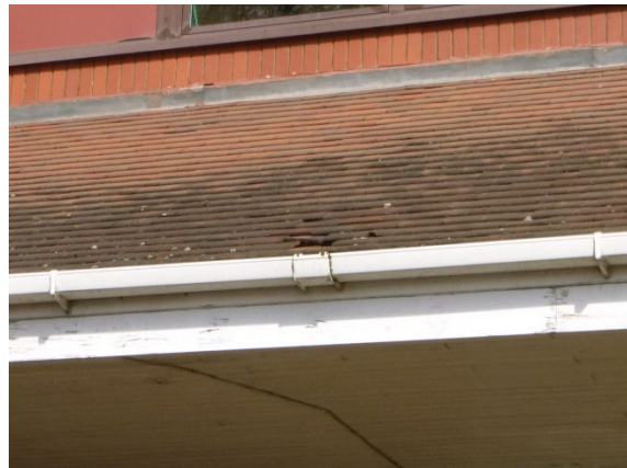
4. Broken roof tile (negligible suitability for roosting bats).
