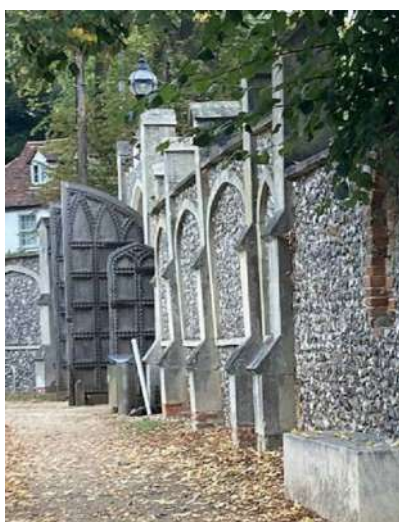
Elevation 2 looking North showing the lean of the wall into the garden
