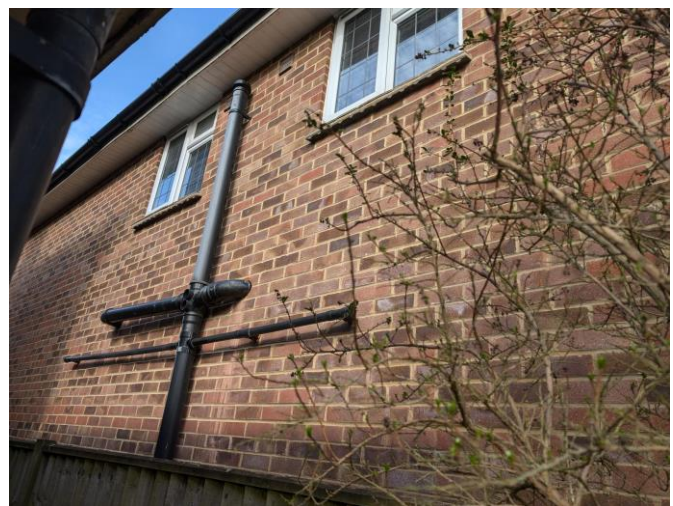
Note the sewerage pipes typical of bathrooms.
