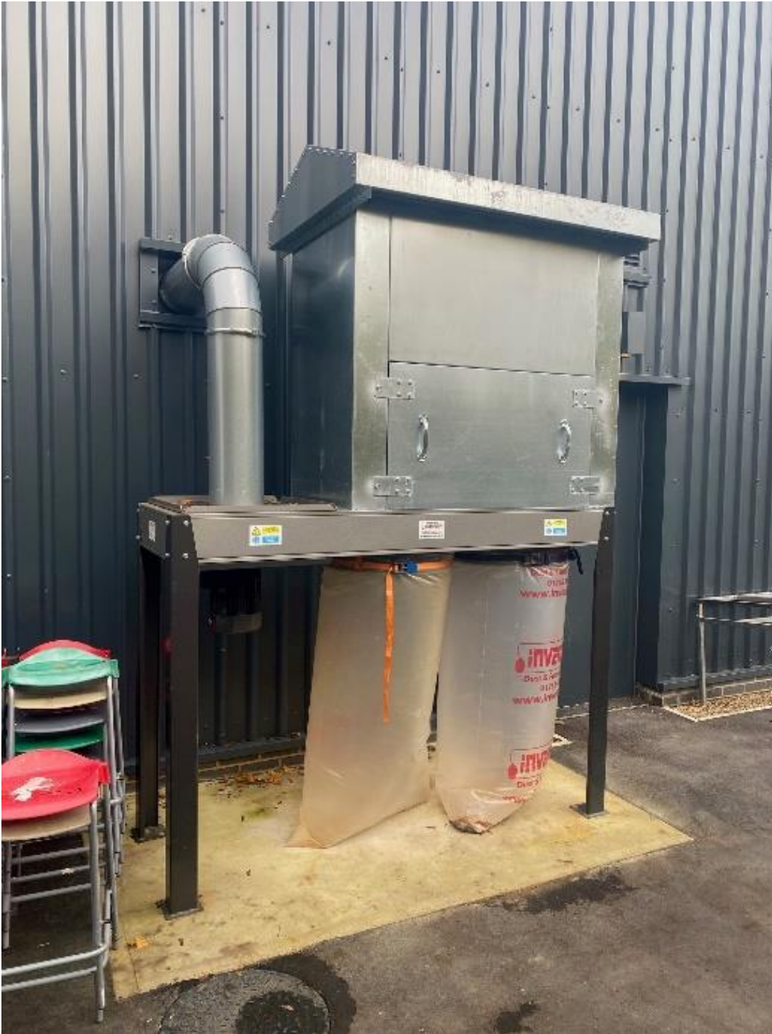
Figure A3-1 External plant unit prior to mitigation
