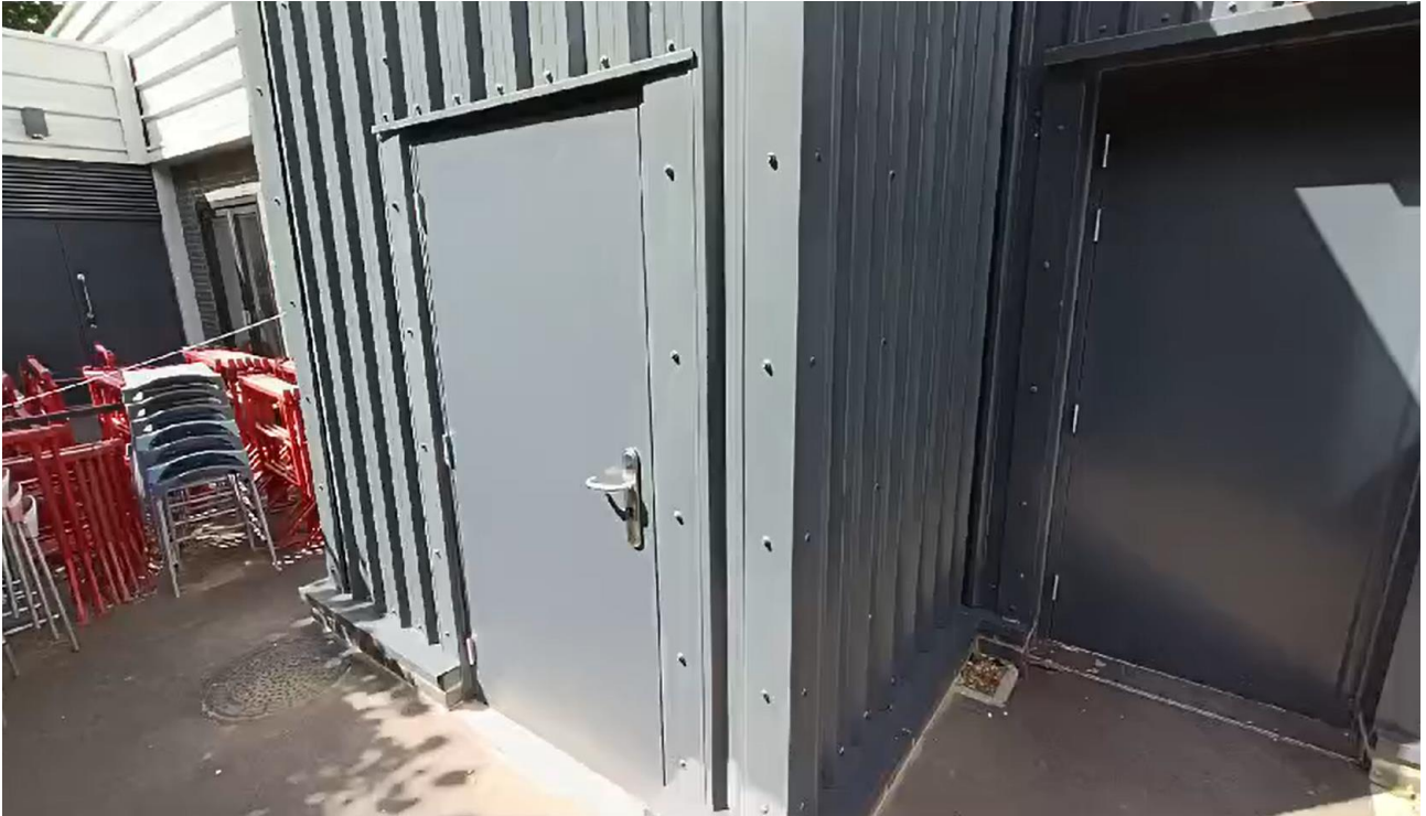
Figure A3-2 External plant unit post mitigation
