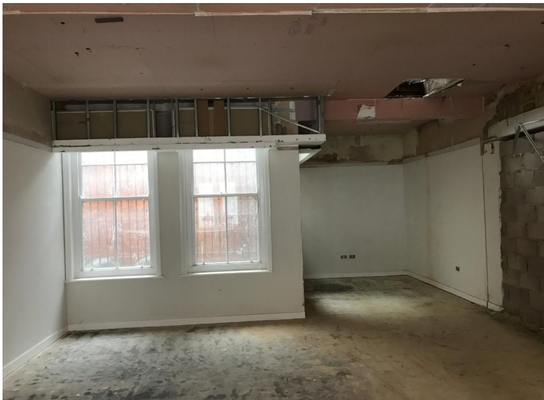
Plate 11. More evidence of previous stripping out and lining at the rear of the building. Again, no stair exists to provide access to the upper floor (note blocked former opening to the historic stair now within the adjacent property) and evidence of the suspended ceilings.
