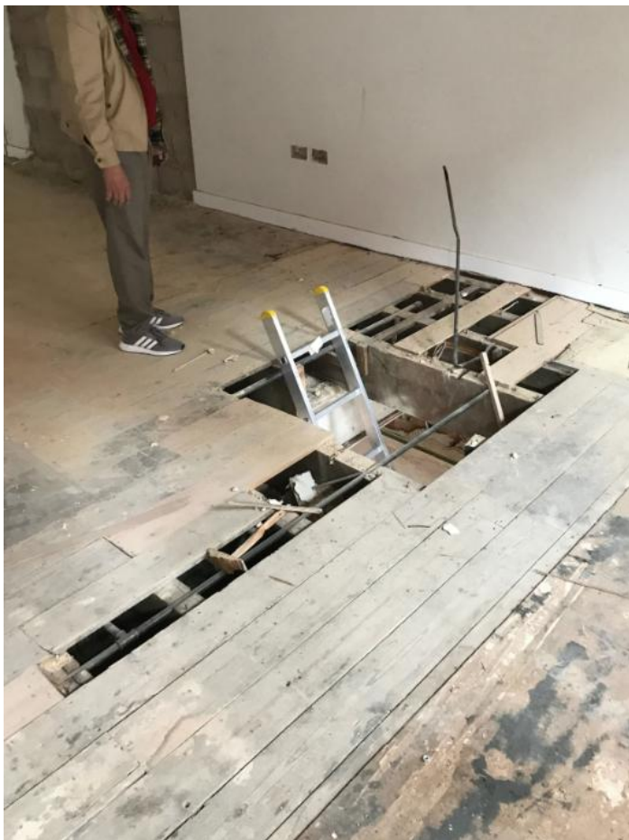
Plate 9. A hole formed to gain access to the upper floors (no stair exists).
