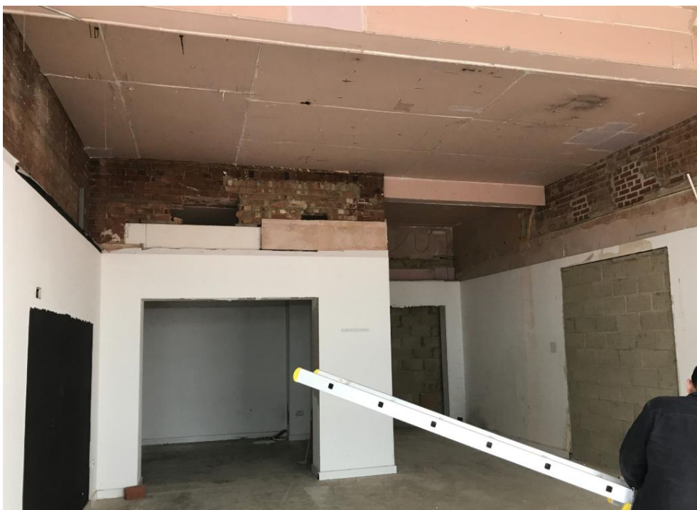
Plate 7. The rear of the ground floor. This is typical of the inherited finish on all floors.
