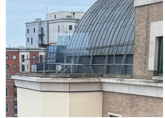
One of the existing railings at fourth floor level to be replaced
