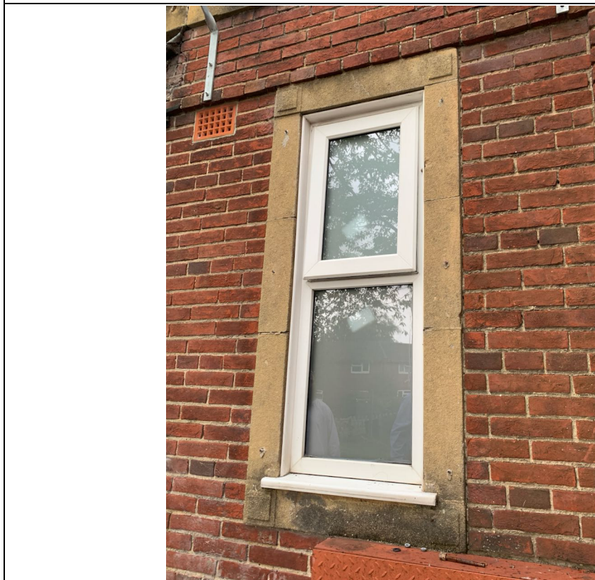
Damage from fixings around a window on the south side of the building August 2021
