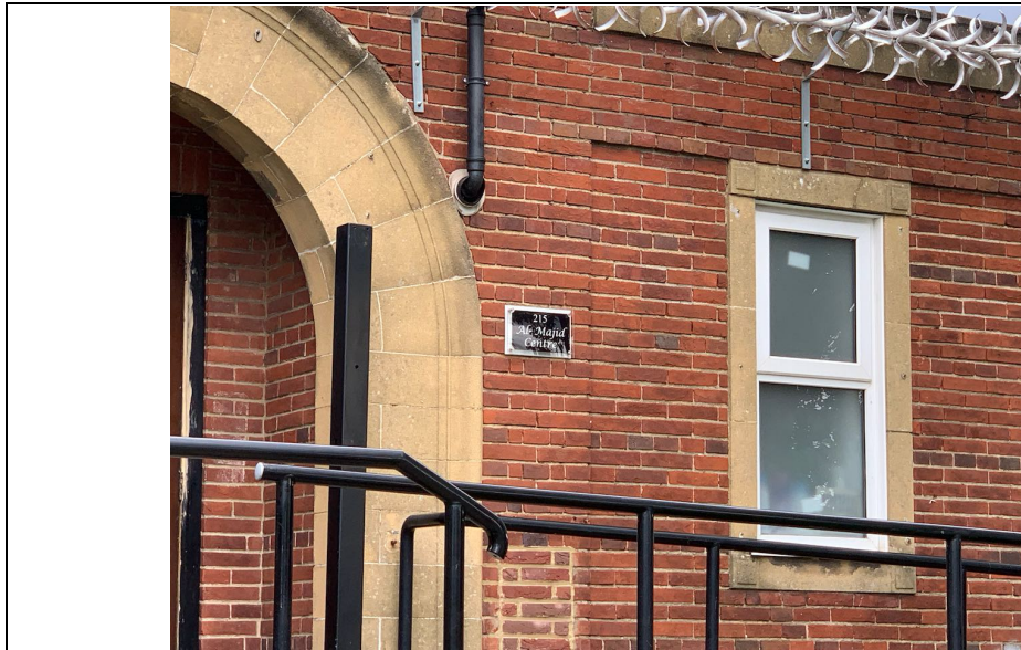
Damage from fixings around the porch and window August 2021
