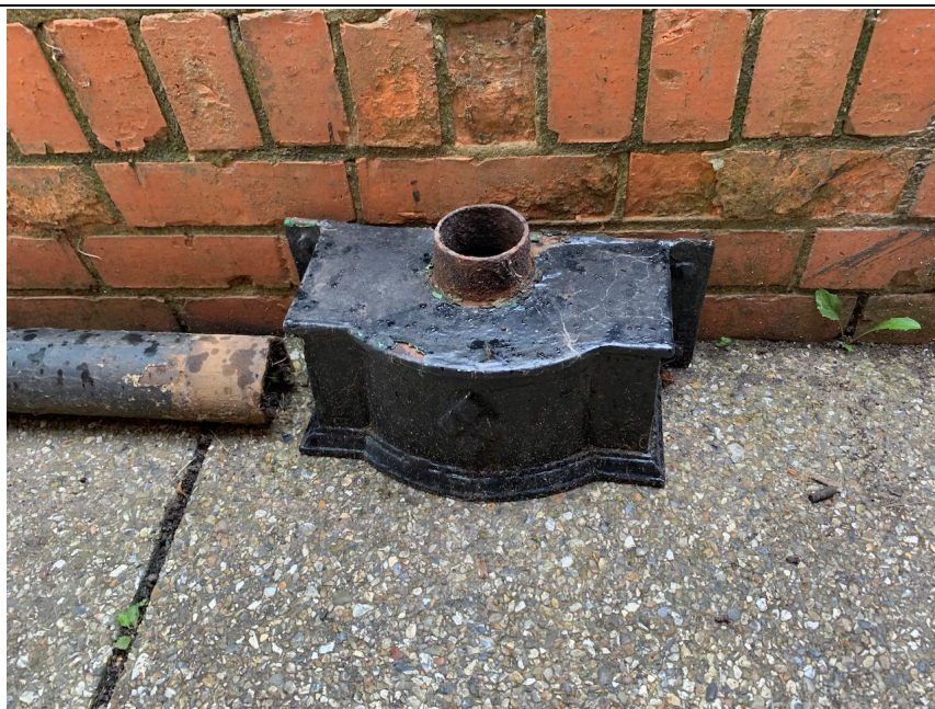
Cast iron hopper and drainpipe August 2021
