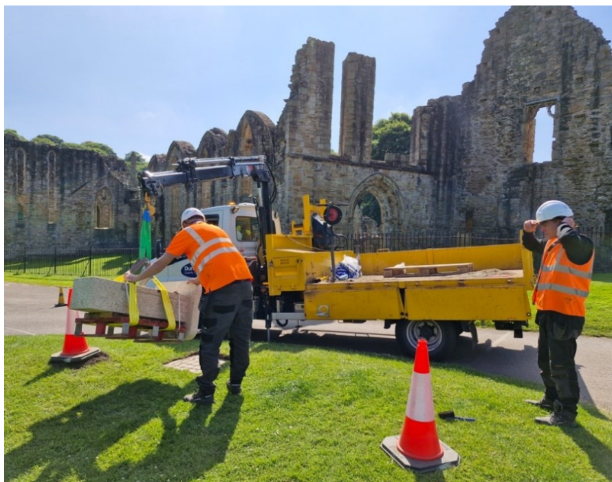
Photo 4.5A – Installation at Finchale Priory near Durham
