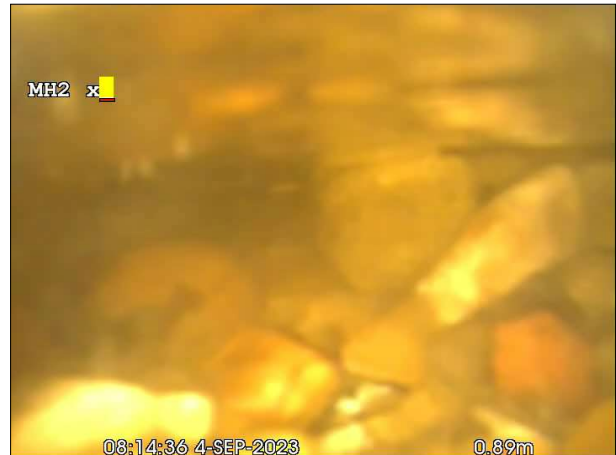
Photo: 1_5a, 00:00:00 0.89m, Debris, 20 % cross-sectional area loss
