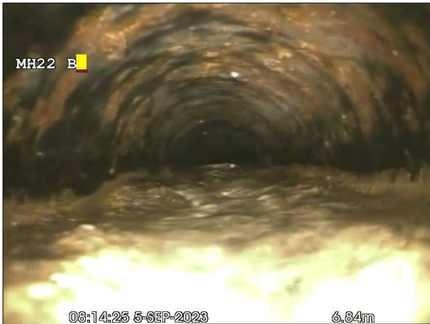
Photo: 284_5a, 00:00:00 6.5m, Debris silt, 50 % cross-sectional area loss, Start,
