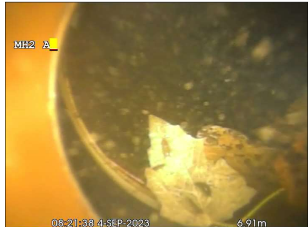
Photo: 33_6a, 00:00:00 7m, Joint displaced. Medium
