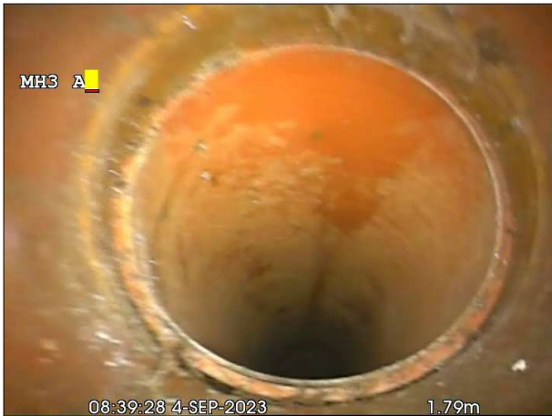
Photo: 70_5a, 00:00:00 1.8m, Joint displaced. Medium
