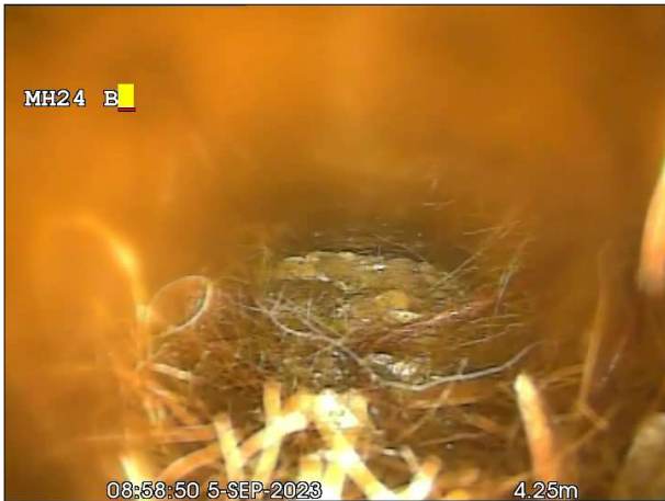
Photo: 344_5a, 00:00:00 4.9m, Debris, 95 % cross-sectional area loss
