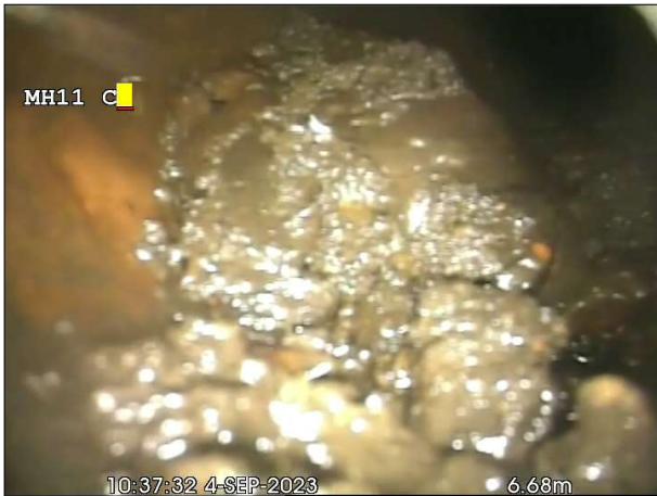
Photo: 174_7a, 00:00:00 6.8m, Survey abandoned, Remark: Unable to pass blockage
