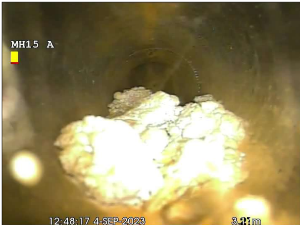
Photo: 219_5a, 00:00:00 3.1m, Debris silt, 10 % cross-sectional area loss
