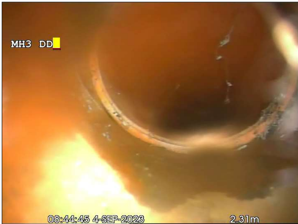
Photo: 8_6a, 00:00:00 2.5m, Joint displaced. Medium
