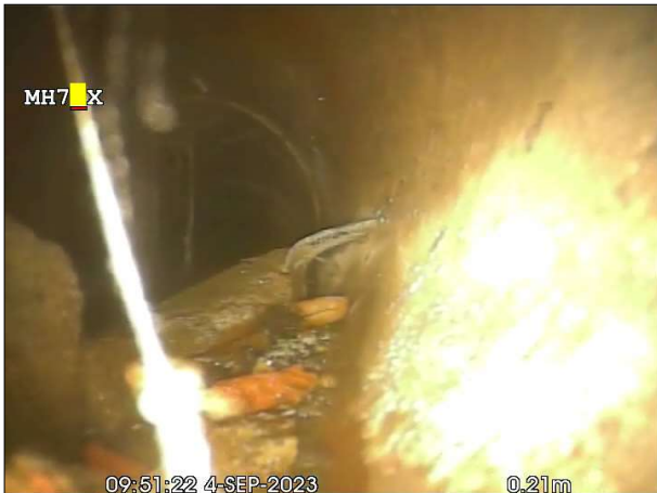
Photo: 15_3a, 00:00:00 0.3m, Debris, 30 % cross-sectional area loss
