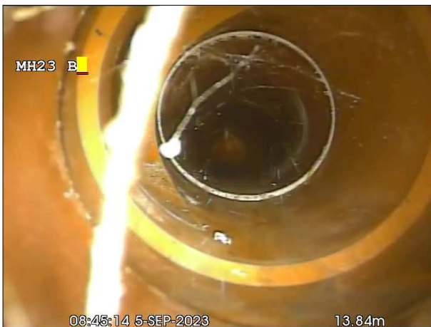
Photo: 323_7a, 00:00:00 13.8m, Joint displaced. Medium
