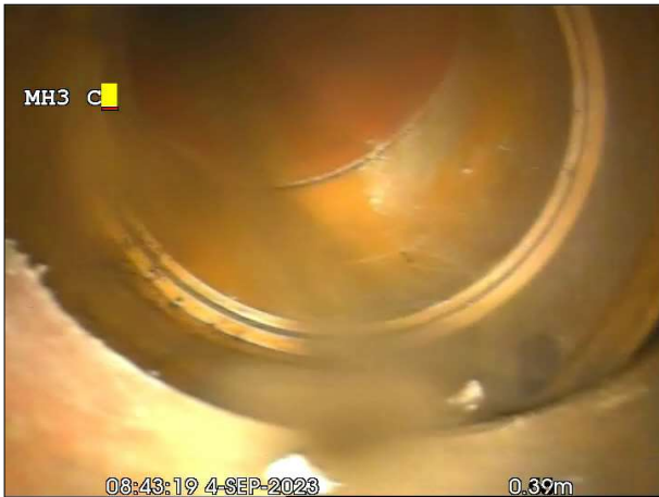
Photo: 84_3a, 00:00:00 0.4m, Joint displaced. Medium
