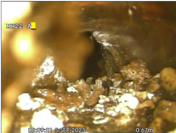
Photo: 278_5a, 00:00:00 0.7m, Debris, 50 % cross-sectional area loss
