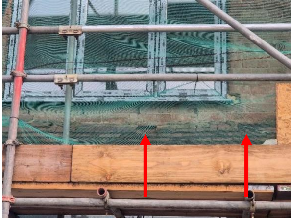
Photograph 16: Missing and lifted tiles on the porch roof on the western elevation of B1.
