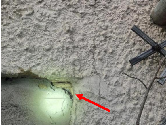
Photograph 12: Gap above a ground floor window on the eastern elevation of B1.
