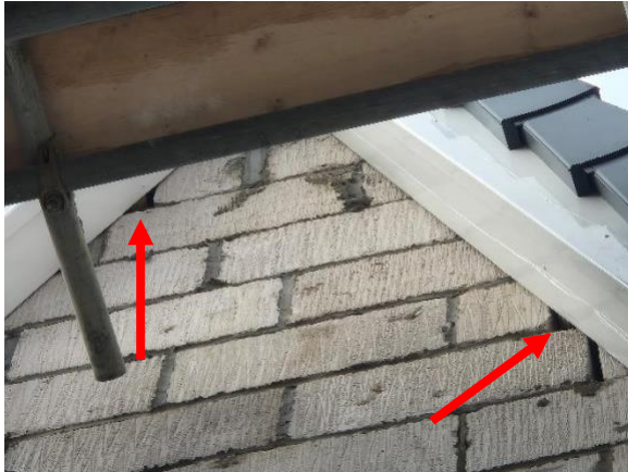
Photograph 10: Gaps in the blockwork on the gable end on the eastern elevation of B1.
