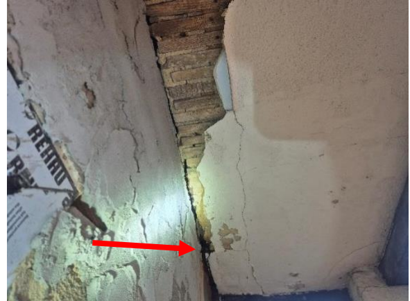
Photograph 17: Damage above the front door on the western elevation of B1.
