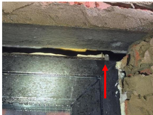
Photograph 15: Gap above a ground floor window on the southern elevation of B1.
