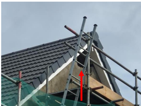
Photograph 14: Gap at the apex on the southern elevation of B1.
