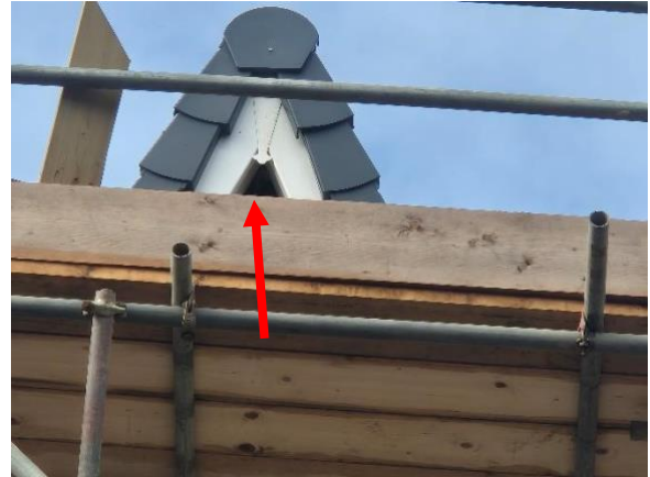
Photograph 11: Gap at the apex of the gable end on the eastern elevation of B1.
