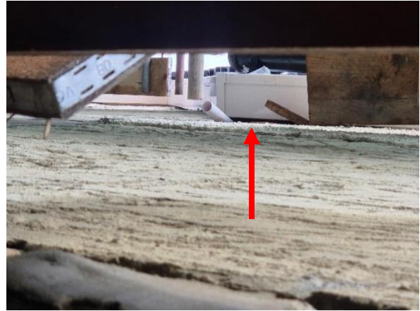
Photograph 13: Gap behind the soffit on the southern elevation of B1.
