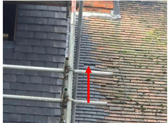
Photograph 9: Missing tile on the eastern elevation of B1.
