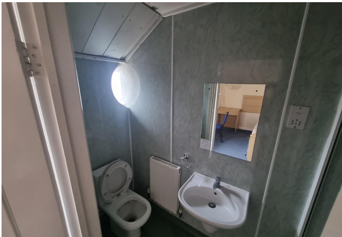
Fig.15: Example of one of six such small post-construction bathrooms located to the east and west sides of the building to the first and ground floors.
