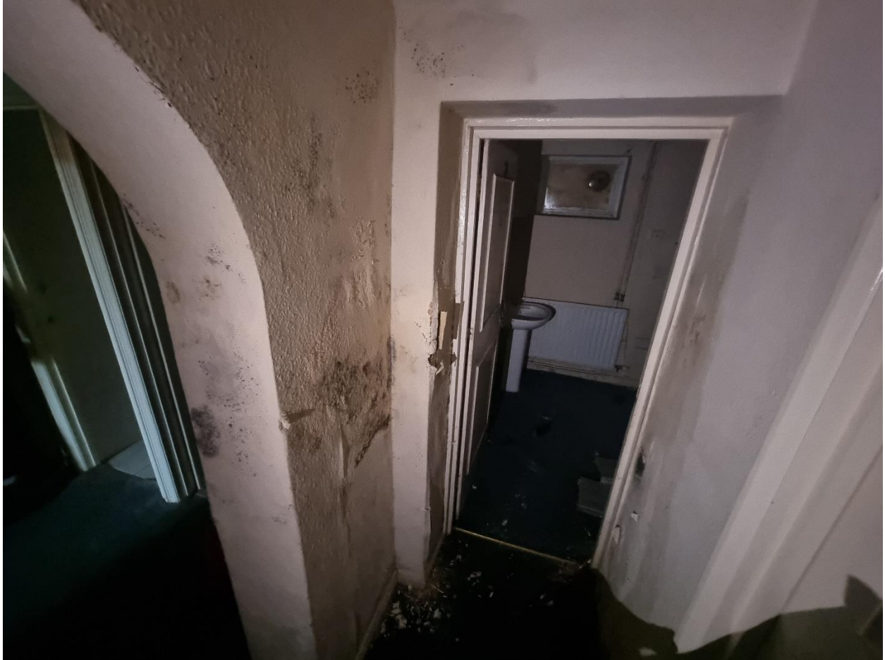
LGF5 – Modern fabric, damp to altered arch opening
