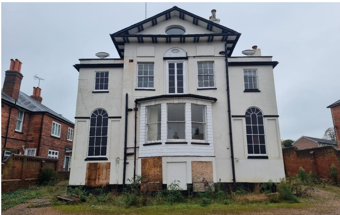
Fig.9: Rear elevation with four blocked up and painted windows (ground floor arches, first floor middle and far left), early/mid-20 th century windows to bay, gable end window altered to fixed pane rather than swivel opening.
