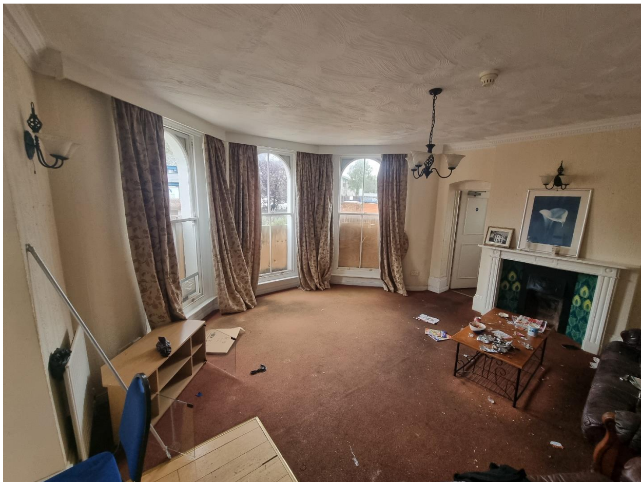
GF2(2) – Mixed context historic and replacement skirting and cornice, c.early 20 th century replacement windows with modern single glazing (non-original but mentioned in 1976 listing)
