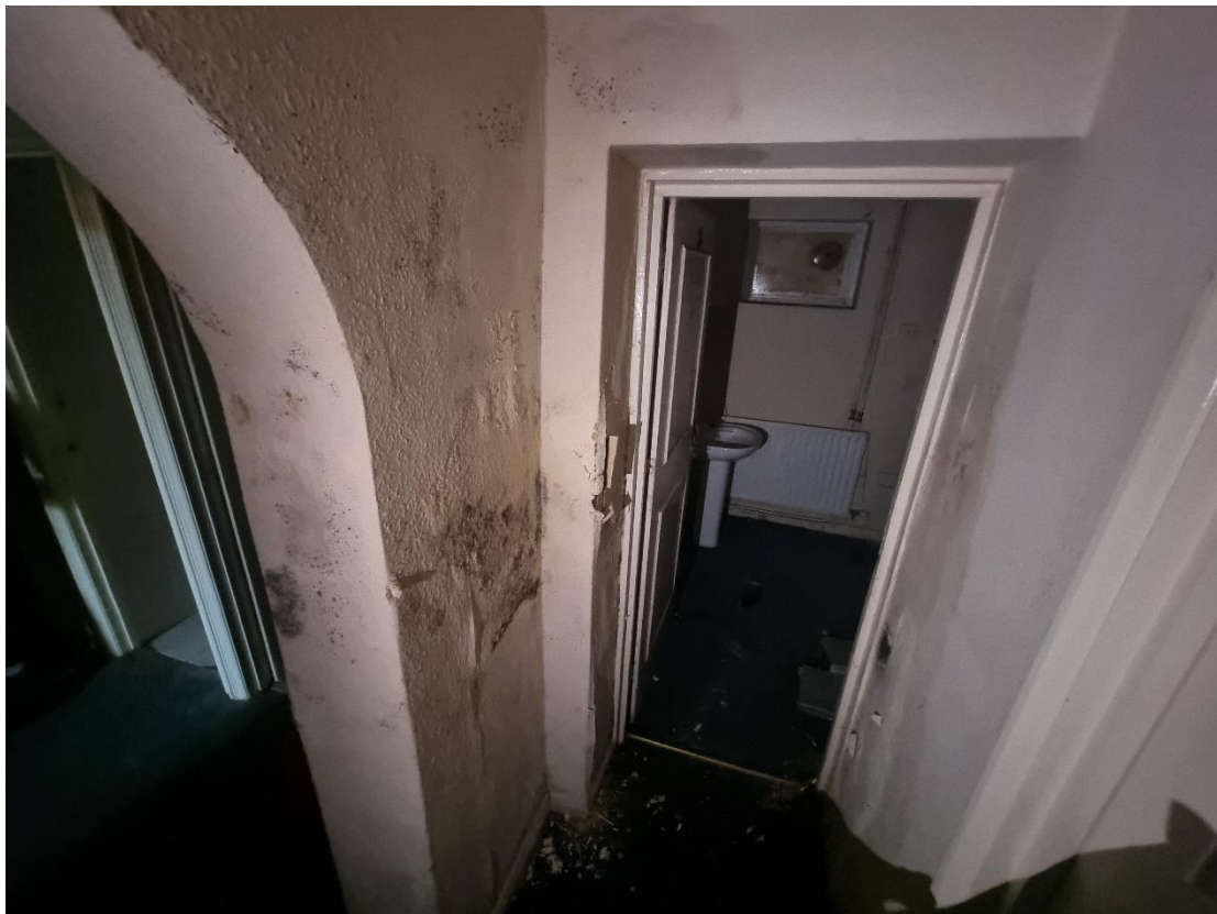
Fig.21: Basement level arch opening to stairwell, looking towards a bedroom to the east side of the building. This floor is in particularly poor condition with damp and damage commonly found and entirely lacking historic fabric.
