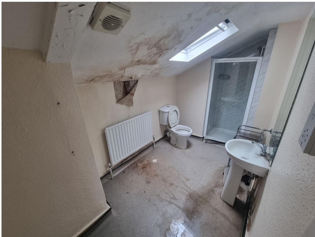
SF5 – Modern fabric, damage caused by ceiling leak
