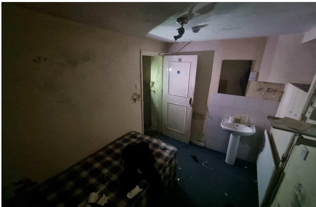
Fig.22: Example of lower ground floor bedroom – low light due to boarded windows and shut-off power during the site visit.
