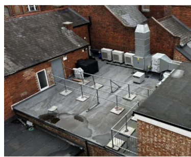
Typical roof mounted AC heat pumps
