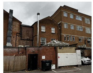
Typical high level kitchen extracts
