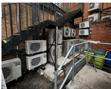
Typical wall mounted AC heat pumps
