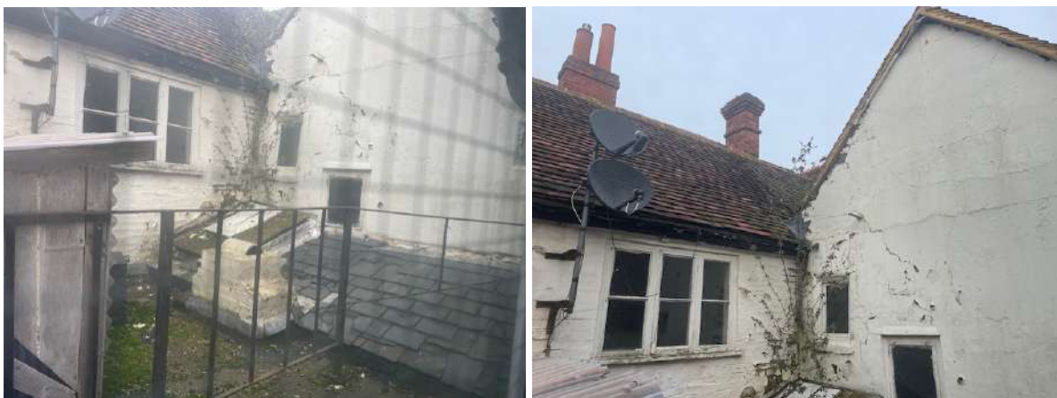
Figure 7: The flat and pitch roof in the courtyard was found to be poor condition; Figure 8: The upper floor elevation walls were found to have hairline cracks in the plaster.
