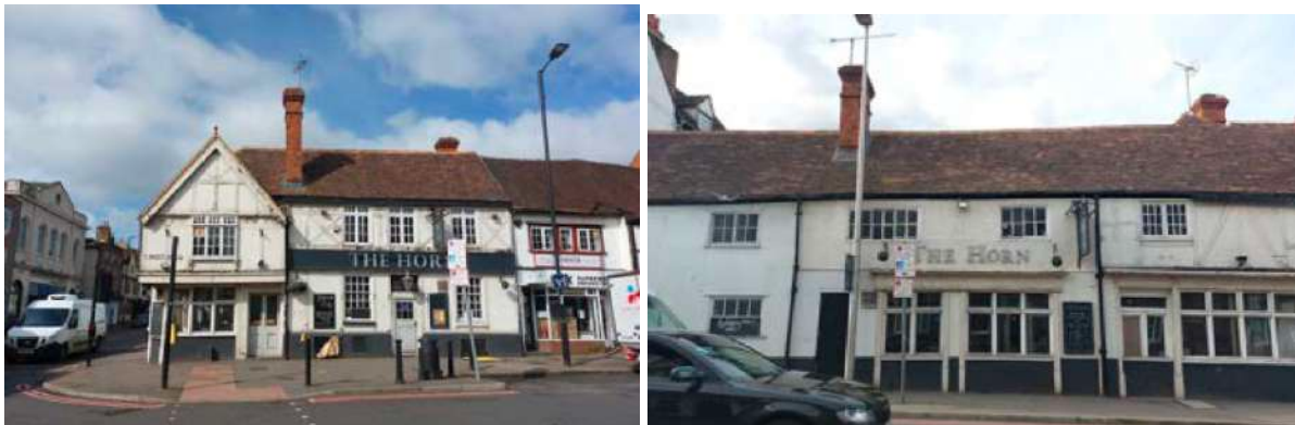
Figure 5: Front Elevation can be confirmed to have partially weathered timber structural members painted in white colour; Figure 6: The Side Elevation showed timber members to have failed.
