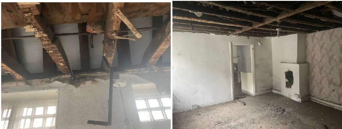
Figure 13: The ceiling joists can be confirmed to have failed and plasterboard ceiling can be confirmed not original; Figure 14: The timber beam supporting the ceiling joists were found to have failed, it would require treatment and strengthening.
