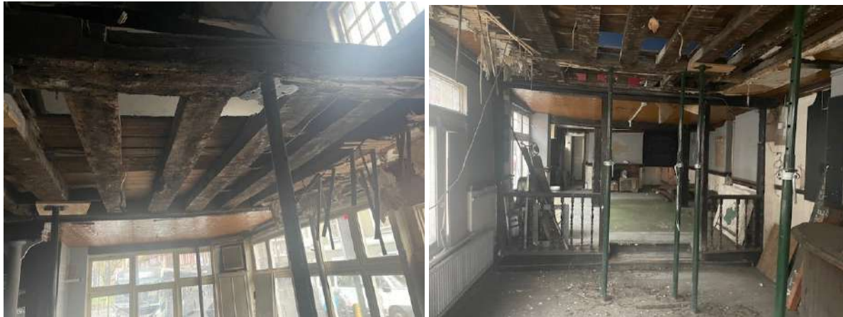
Figure 21: The first floor joists were found to be manifested as well as failed structurally; Figure 22: The temporary support in place was found to be acceptable.
