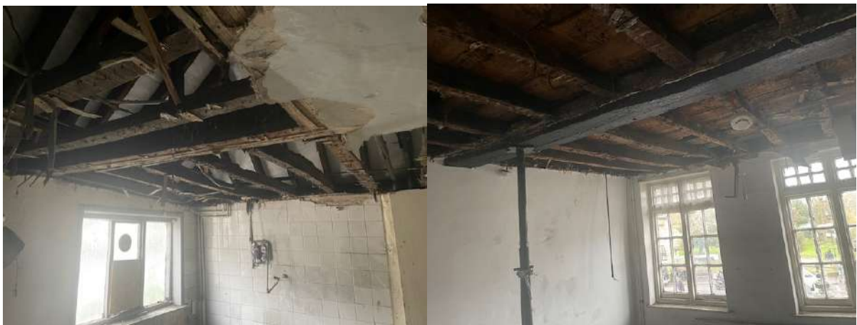
Figure 11: The ceiling joists can be confirmed to have failed and plasterboard ceiling can be confirmed not original; Figure 12: The timber beam supporting the ceiling joists were found to have failed, it would require restoration and strengthening.
