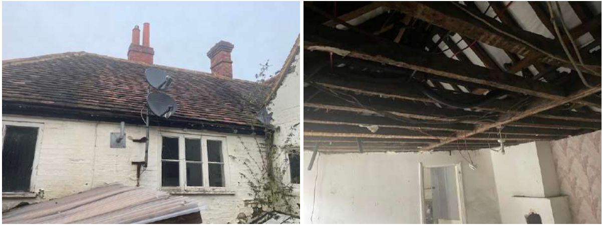
Figure 9: The rear ridge line along with wall above courtyard was found to be adequate; Figure 10: The rafters had a history of deflection, manifestation and deflection including the ceiling joists.
