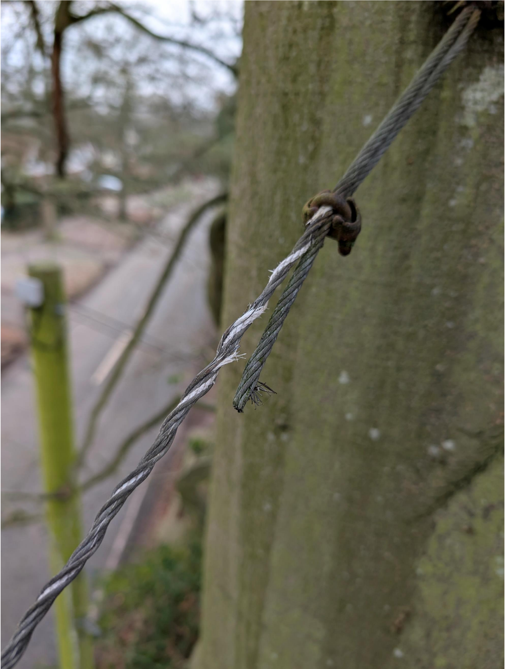
B.3 - Image of cable deterioration near central stem attachment point.
