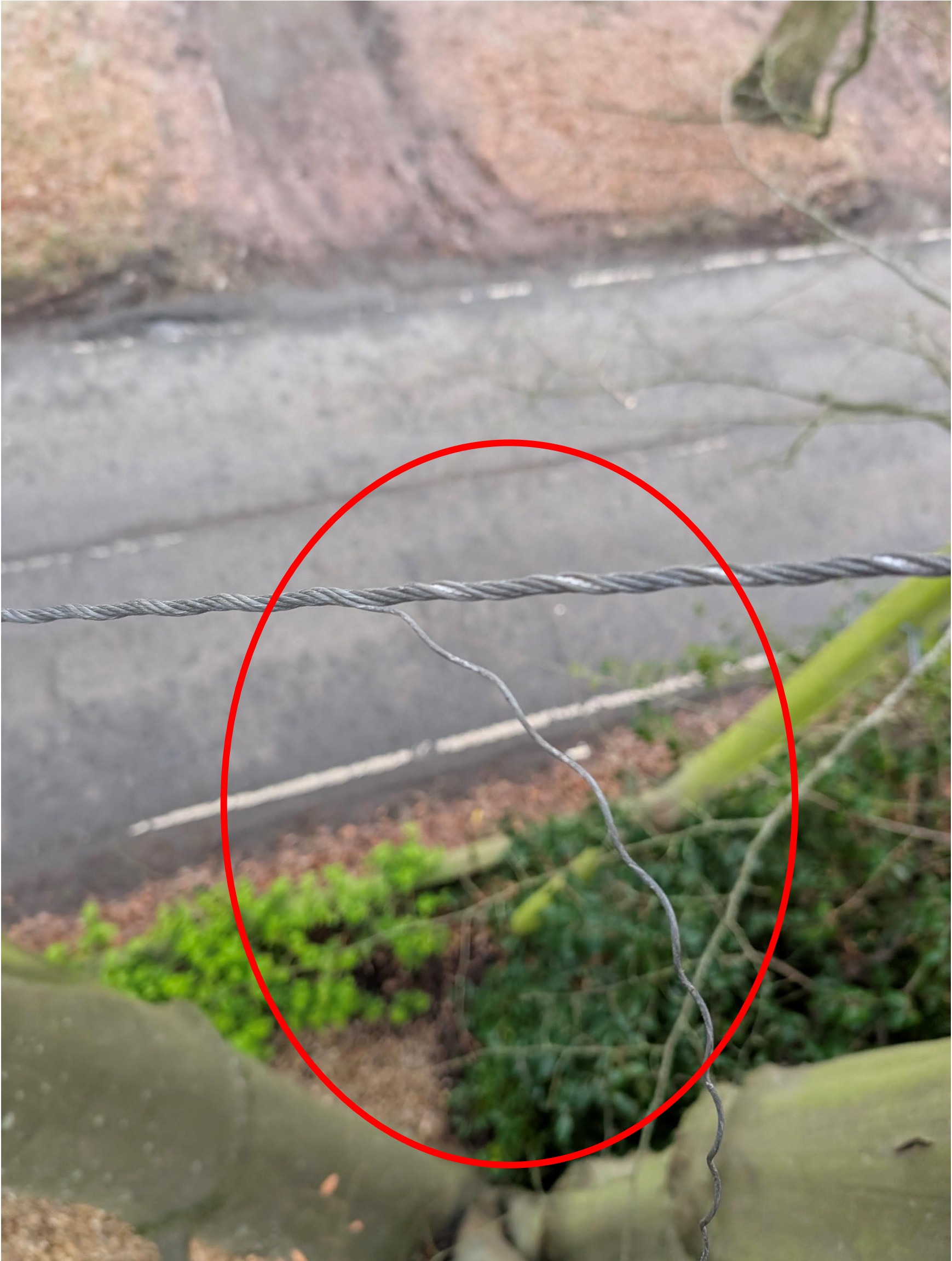
B.2 – Image of installed cable bracing with single broken cable.
