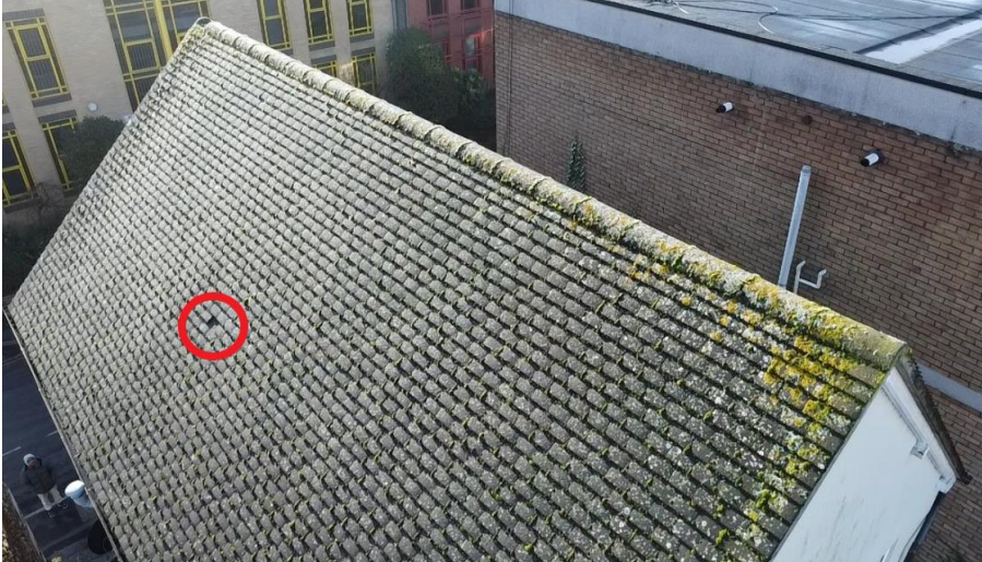
Figure 8: The missing tile on the east roof slope, highlighted in red
