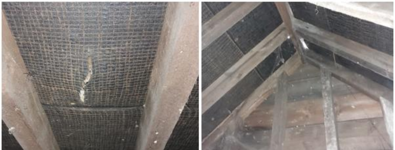
Figure 5: A tear in the roofing membrane and light entering through the south gable apex
