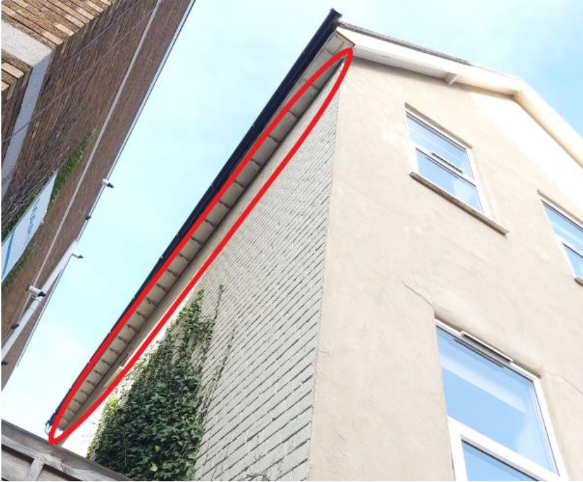
Figure 6: Gap between the soffit and the wall on the west elevation, highlighted in red
