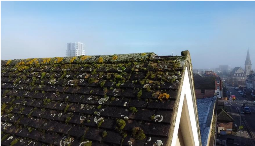
Figure 7: The roof from the south side, showing the missing ridge tile above the gable apex
